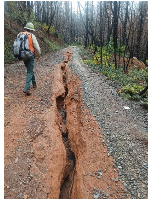
Photo 2. Road surface runoff resulting in gully erosion and subsequent sediment delivery to a perennial watercourse downslope.
