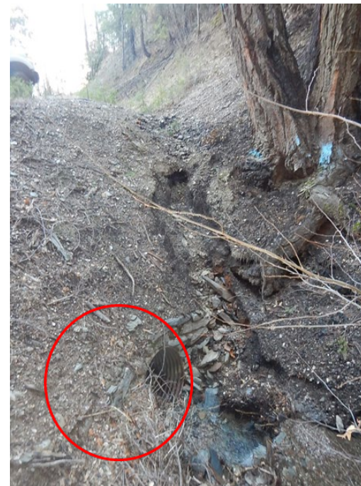
Photo 11. Fill slope erosion and sediment delivery above an intermittent watercourse crossing. Culvert inlet is circled in red.
