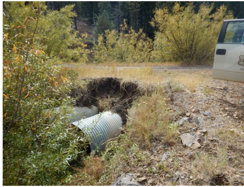
Photo 8. Evident scour above perennial watercourse crossing 'double-barreled' inlets.
