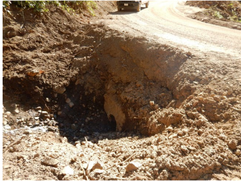
Photo 7. Partially plugged (undersized) ephemeral watercourse crossing inlet.
