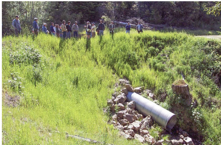
Photo 3. Rock armor placed around a culvert outlet to dissipate erosive forces.
