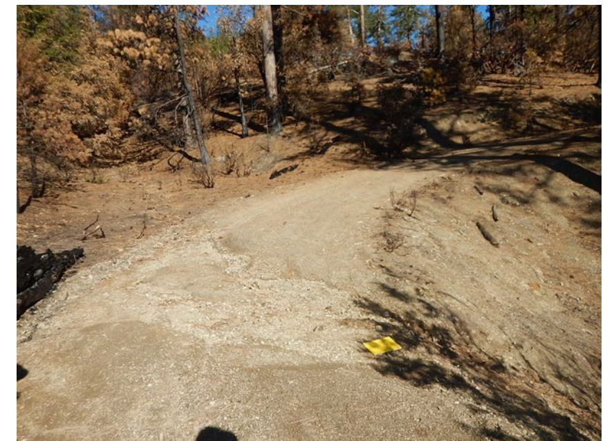
Photo 12. Road surface runoff resulting in erosion and sediment delivery to an ephemeral watercourse downslope. Yellow notebook for size reference.
