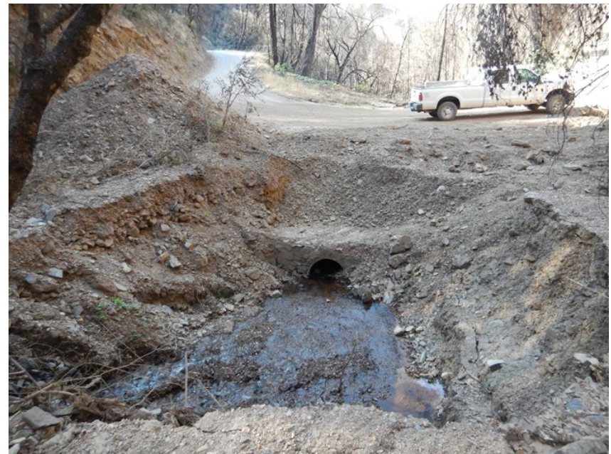
Photo 16. Undersized ephemeral watercourse crossing inlet; unarmored fill slope above the crossing.
