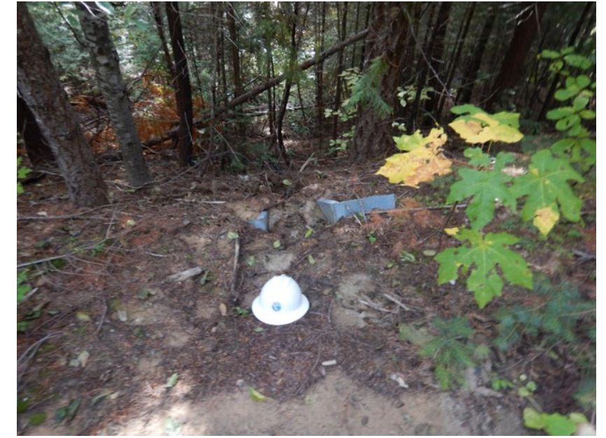
Photo 9. Plugged overside drain and subsequent sediment delivery to a perennial watercourse at the bottom of this slope.
