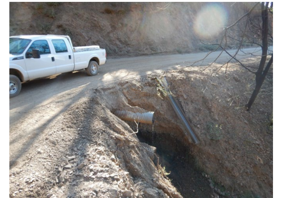
Photo 6. Ephemeral watercourse crossing outlet with a 'shot-gunned' culvert causing road fill scour.
