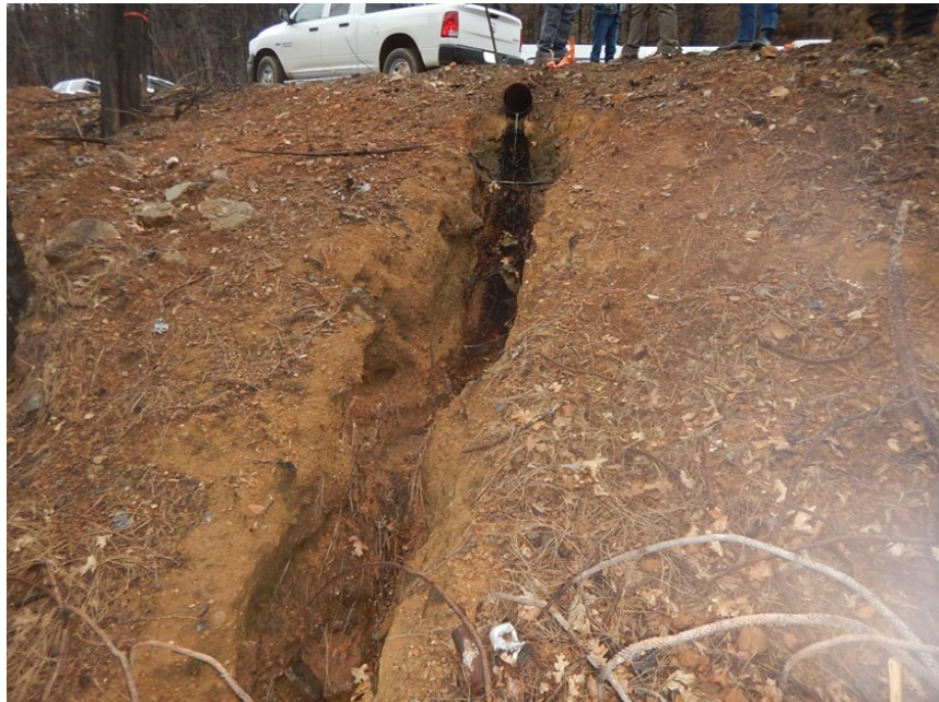
Photo 13. Road fill erosion resulting from a lack of armoring below a drainage ditch relief culvert outlet.
