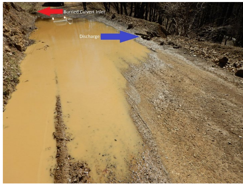
Photo 14. Road surface ponding due to a buried drainage culvert (red arrow) with subsequent discharge over the fill slope (blue arrow) into an intermittent watercourse downslope.
