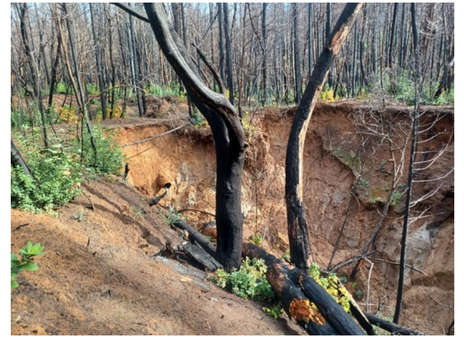
Photo 3. Road fill failure due to a plugged culvert inlet and overtopping. Perennial watercourse crossing outlet circled in red.
