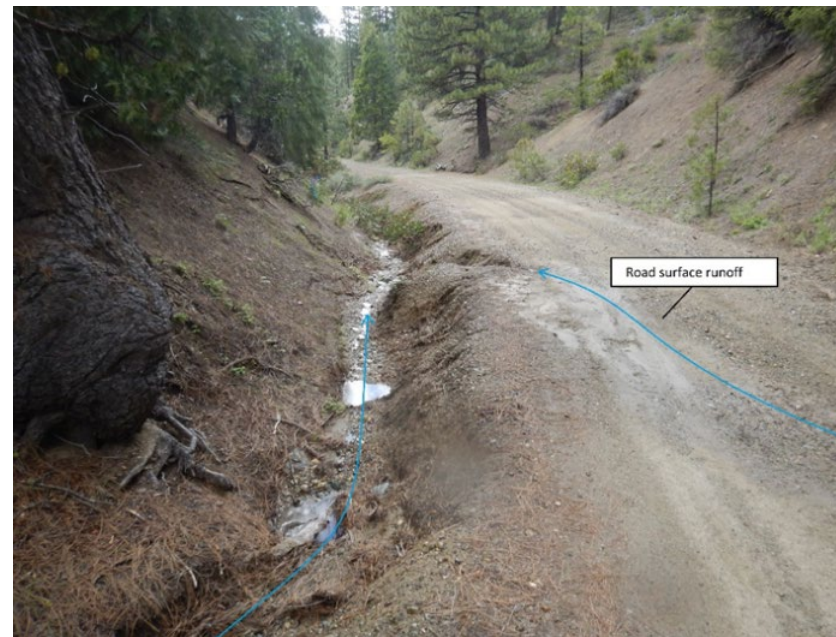
Photo 5. Road surface runoff resulting in erosion and sediment delivery to a drainage ditch which discharges to a perennial watercourse downslope.
