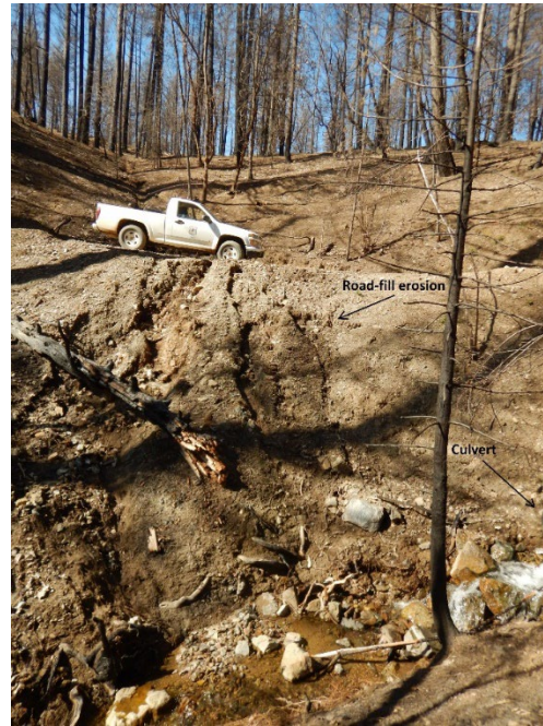
Photo 1. Roadfill erosion discharging sediment below an intermittent watercourse crossing. Edge of culvert outlet circled in red.
