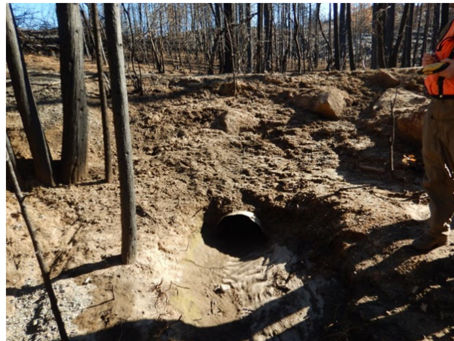
Photo 10. Partially plugged ephemeral watercourse crossing outlet with fill slope erosion above.
