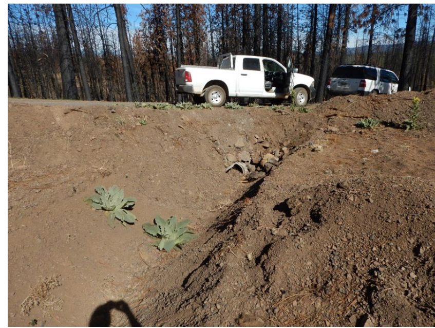
Photo 17. Undersized and partially crushed ephemeral watercourse crossing inlet; unarmored fill slope above the crossing.
