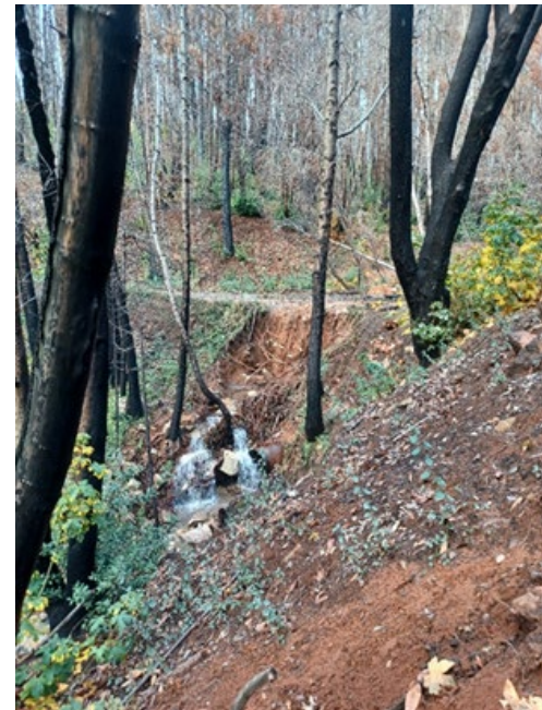
Photo 4. Another road fill failure due to a plugged culvert inlet and overtopping. Perennial watercourse crossing outlet circled in red.
