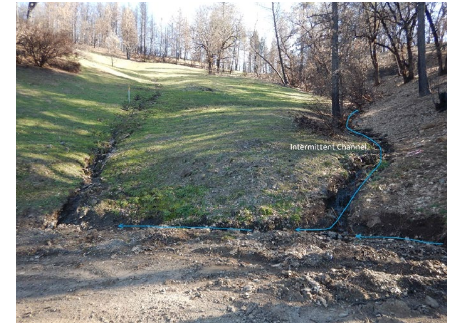
Photo 18. An intermittent watercourse intercepts and diverts into a roadside drainage ditch. Notice the erosion on the hillslope adjacent to the intermittent channel; may be caused from road interaction upslope.
