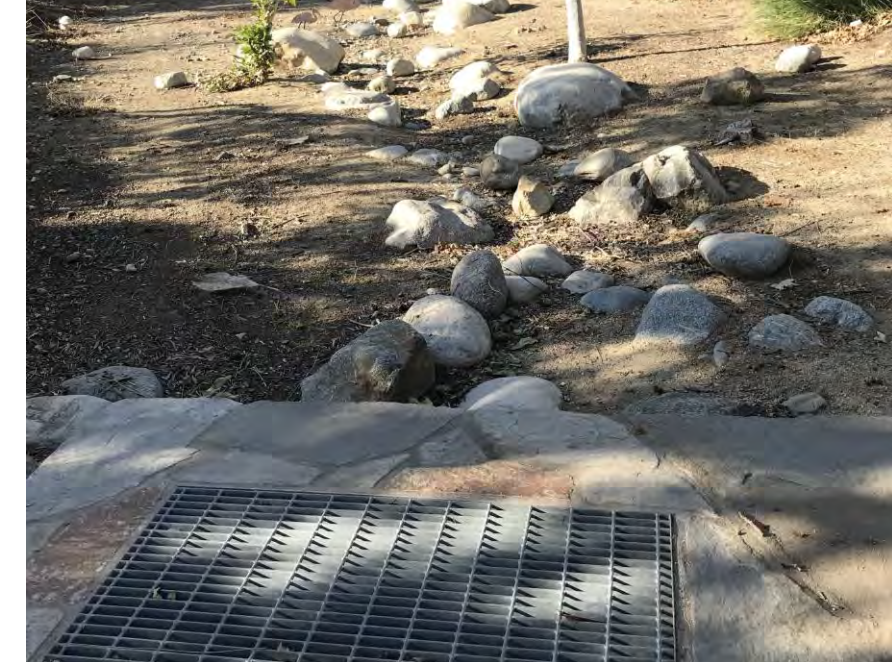
Close Up of Existing Grate Inlet (Circled in Red to Left) from Natural Channel to SD (from SE looking NW)
