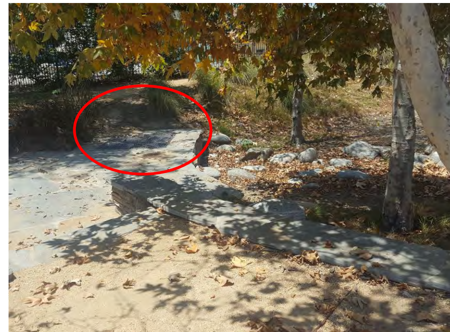
Existing Drainage Basin and Storm Drain Inlet at South End of Park (from NE looking SW)
