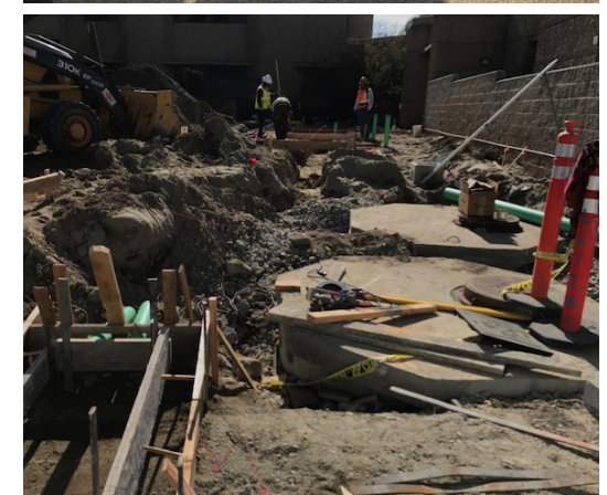
Stormwater Capture in the City of Duarte
