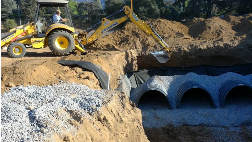
Stormwater Infiltration in City of Bradbury
