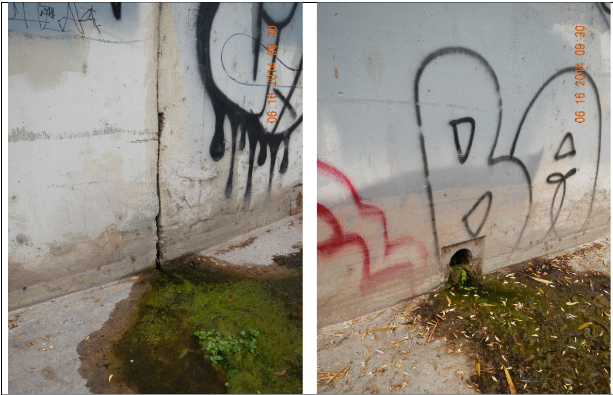
Figure 6-42. Photos of groundwater seepage into Franklin Creek. Photo Credit: Central Coast Water Board staff June 16, 2014.
