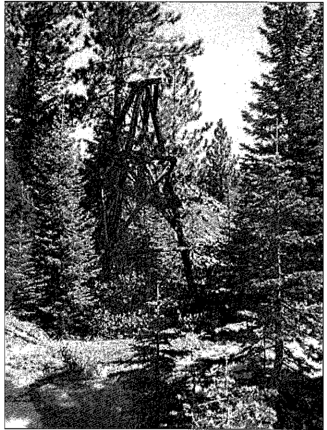
22. Photo of a tower structure for the former aerial tramway that moved supplies and materials between the Walker Mine and Quincy. Shotcrete-lined diversion ditch in the foreground.
