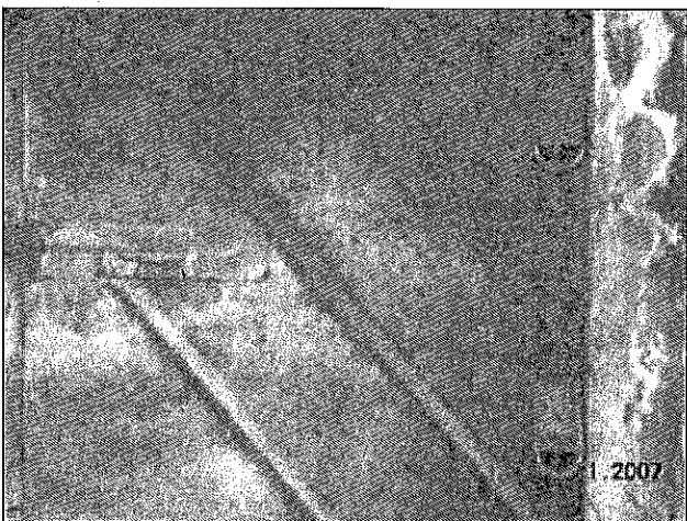
15. Close-up view showing numerous bullet holes in the portal door. The portal access is repeatedly vandalized. Successful entry has been limited.
