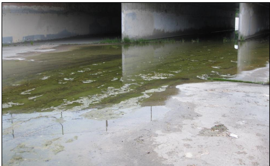
Typical Dry Weather Flow Showing Algal Growth
