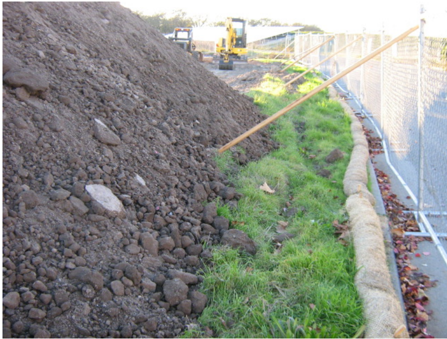
Photograph 7: View showing straw wattle BMPs implemented along the majority of the project site boundary
