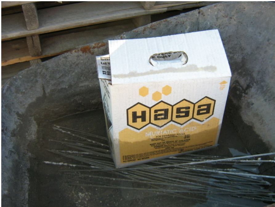
Photograph 2: Container of muriatic acid which was stored in several inches of standing water
