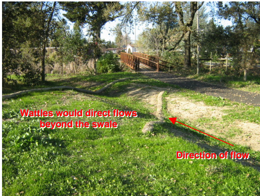
Photograph 16: Straw wattles were not installed to adequately dissipate flow velocity in the swale
