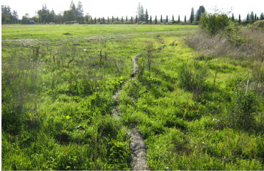
Photograph 15: Straw wattles were badly deteriorated and were no longer necessary or protective of the adjacent wetland (located to the right of photograph)
