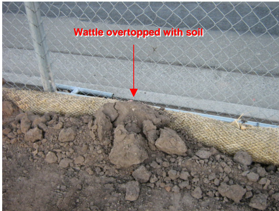
Photograph 11: View showing soil that had overtopped the straw wattle BMP
