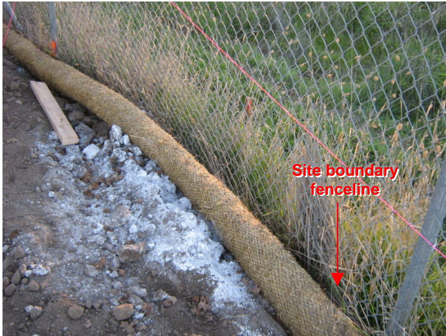
Photograph 5: Lime spillage and/or over-application was observed along the construction site boundary
