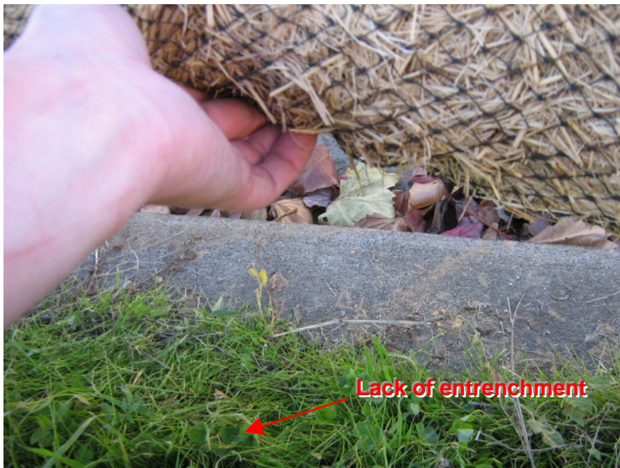
Photograph 8: Straw wattle BMPs were not properly entrenched in the ground to retain sediment
