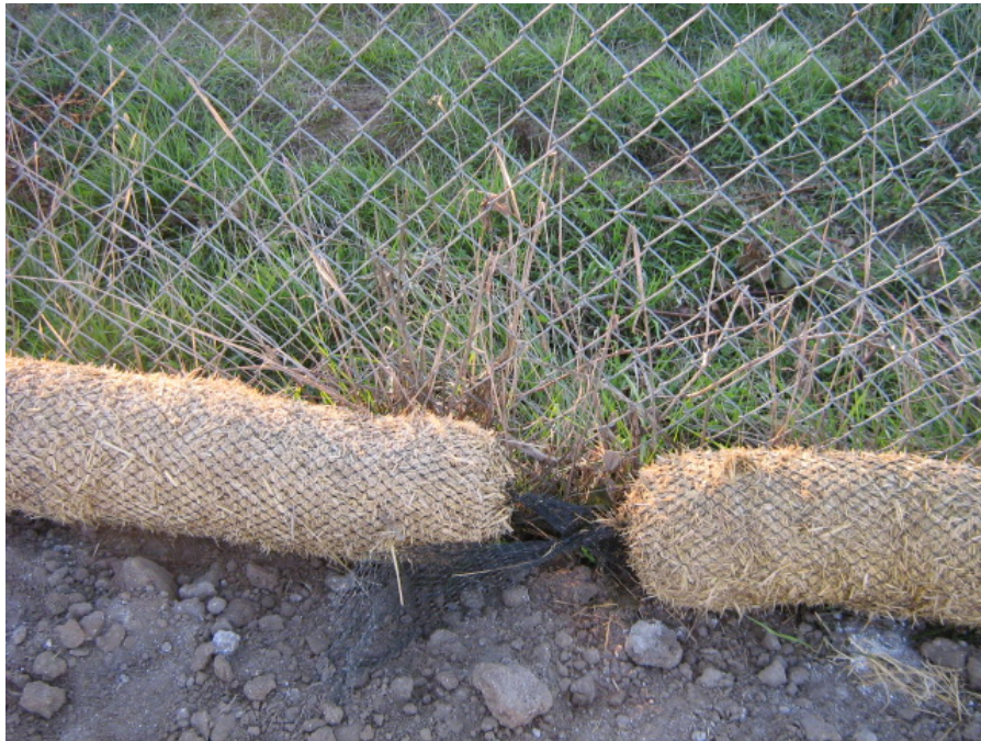
Photograph 9: View of gaps between the lengths of straw wattle BMPs
