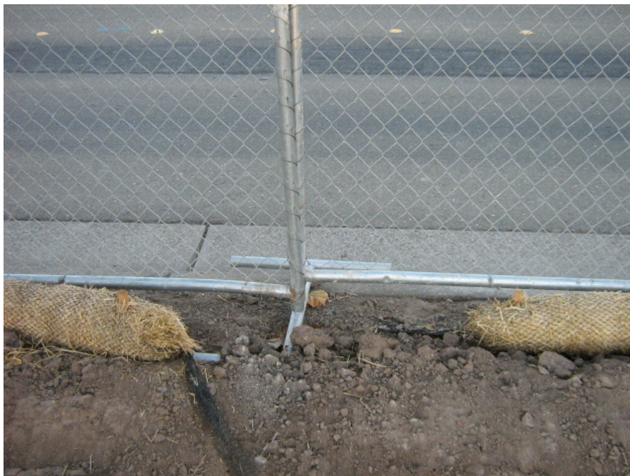
Photograph 10: Additional gaps between the straw wattle BMPs
