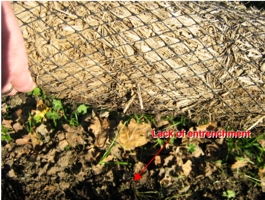
Photograph 14: Straw wattle BMPs were not properly entrenched in the ground to retain sediment
