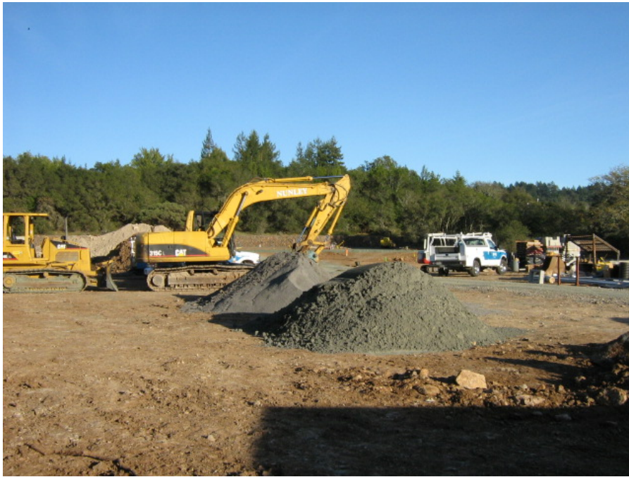
Photograph 1: View of material storage and staging area located in the central portion of the project site
