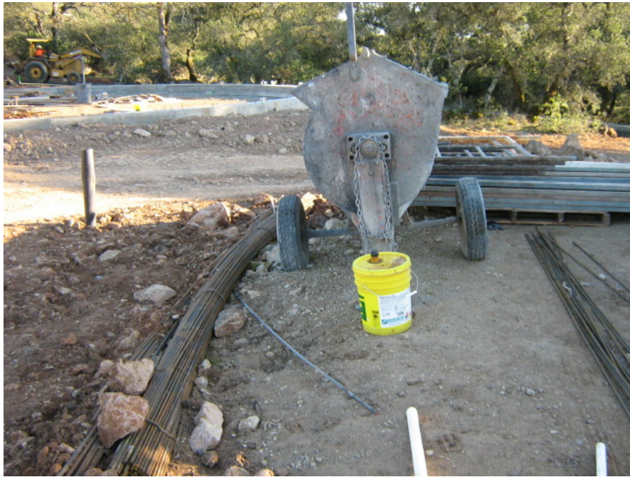
Photograph 3: A container of concrete form release chemical was stored where it could be knocked over and released into the environment
