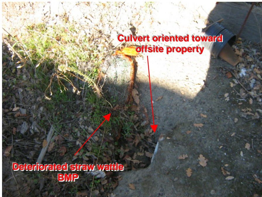
Photograph 22: Close-up view of culvert and associated straw wattle in need of maintenance
