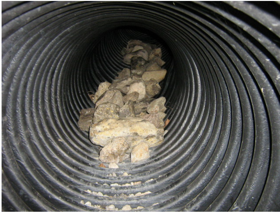
Photograph 19: View of rock and debris near the terminus of the culvert pipe outfall
