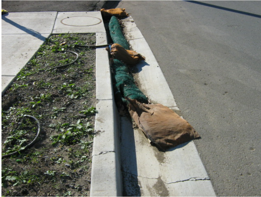
Photograph 3: Sediment transported to the curb and gutter flow-line
