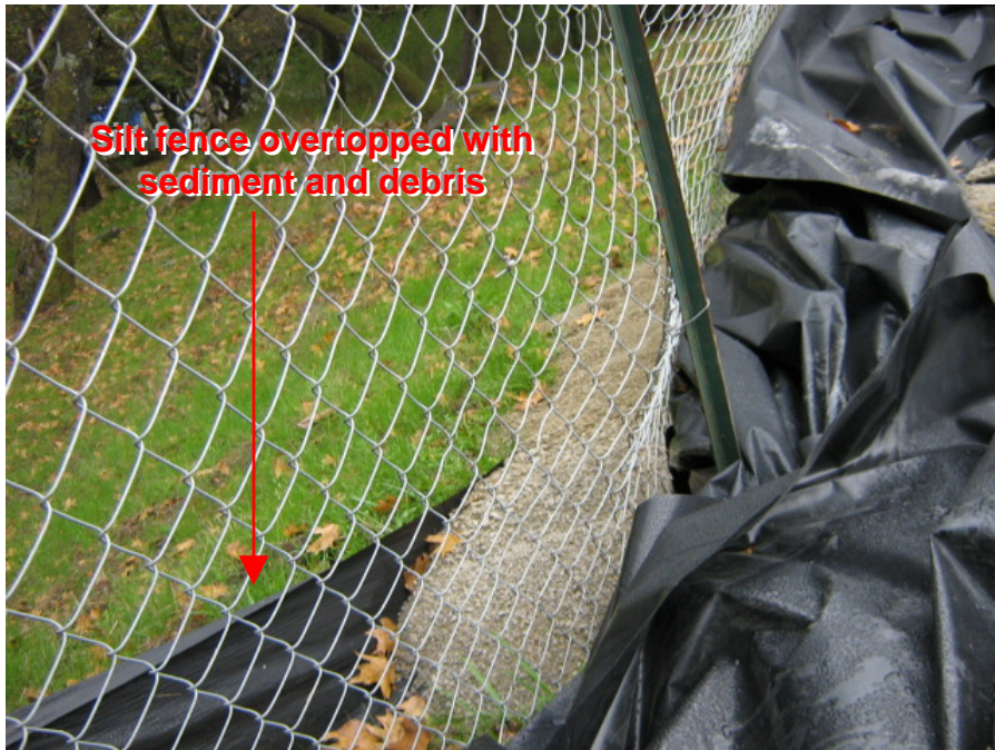
Photograph 12: Unconsolidated material had overtopped the perimeter control silt fence and had been pushed beyond the construction site boundary
