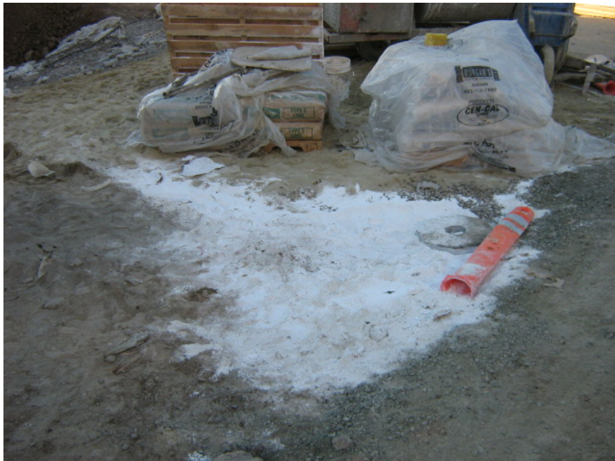
Photograph 8: Lime spillage was present where it could be exposed to storm water contact
