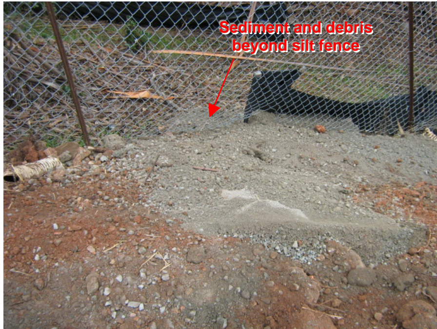
Photograph 13: Sediment transported beyond a section of silt fence located adjacent to the area shown in Photograph 12
