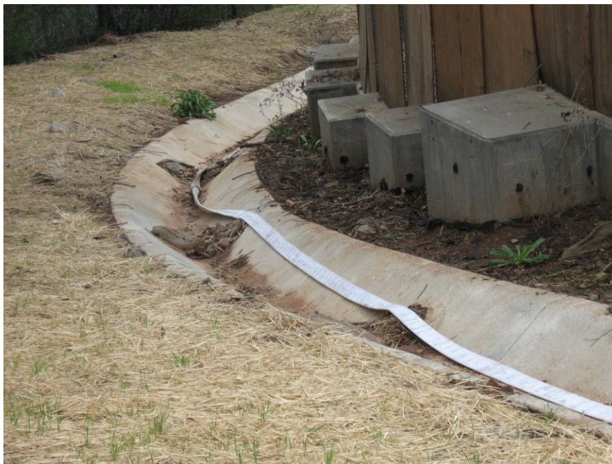
Photograph 16: View of sediment and debris in the brow ditch prior to the flow caused by the leaking fire hose
