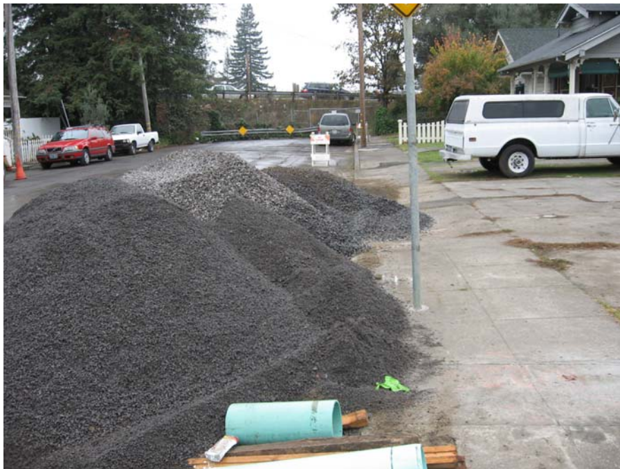
Photograph 18: Placement of material stockpiles in the curb and gutter flow-line and without BMPs
