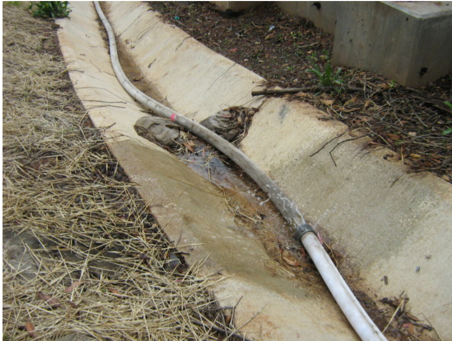
Photograph 15: An actively leaking fire hose, which was connected to a nearby fire hydrant, was placed in the concrete-lined brow ditch
