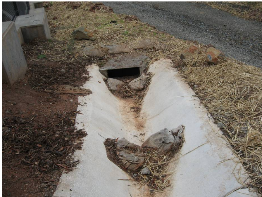
Photograph 14: View of sand bags in the concrete-lined brow ditch which were in need of maintenance
