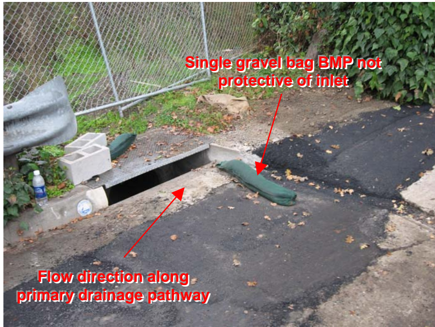
Photograph 19: Inlet protection BMPs were not adequately implemented at the receiving inlet located down-gradient of the material stockpiles shown in the previous photograph
