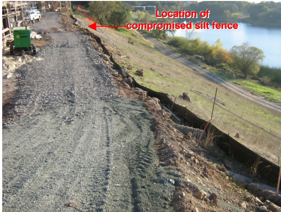
Photograph 5: View depicting location of compromised silt fence and down-gradient waterbody
