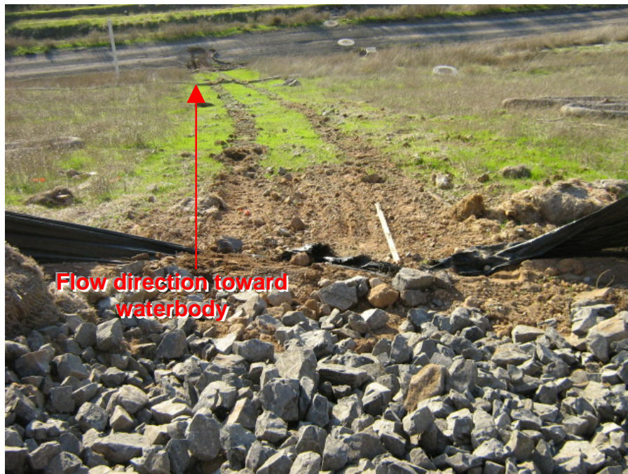
Photograph 6: Length of silt fence compromised by track equipment
