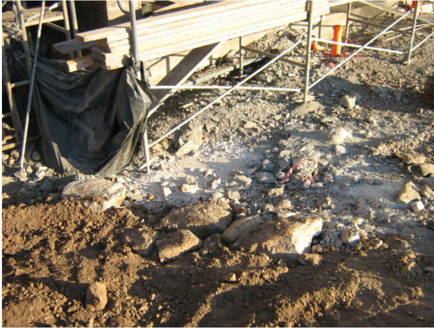
Photograph 9: Spillage of a grout or concrete material was observed in the active building construction area
