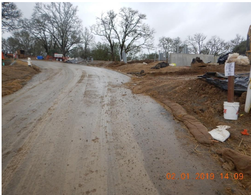
Figure 32. Sediment control BMPs observed do not effectively contain soil within the active construction area.
