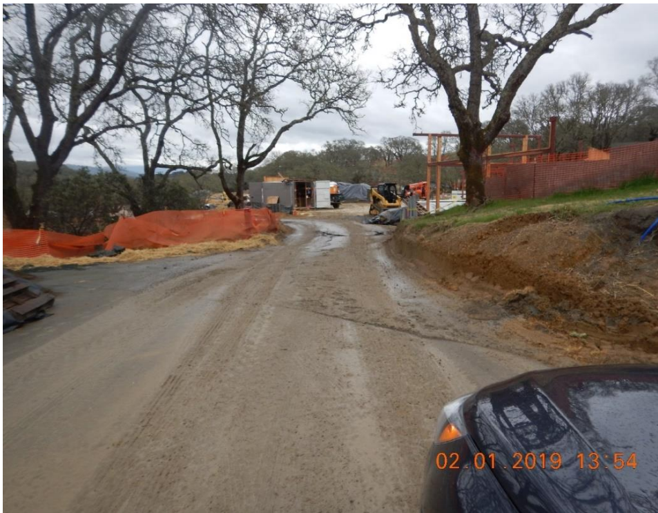
Figure 34. The cut slope adjacent to the roadway lacks erosion or sediment control measures either on the slope or at its toe.
