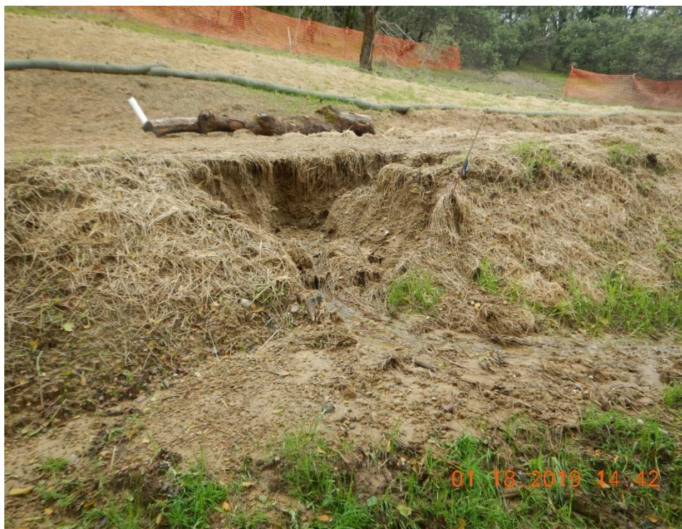
Figure 23. Ineffective erosion and sediment controls on slope resulting in bank failure and evidence of sediment transport in the foreground.
