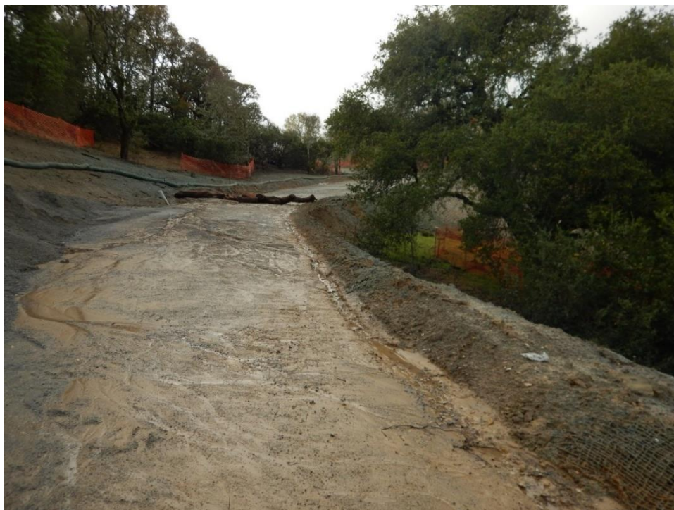
Figure 13. Road segment with adjacent unprotected slope and signs of uncontrolled runoff.
