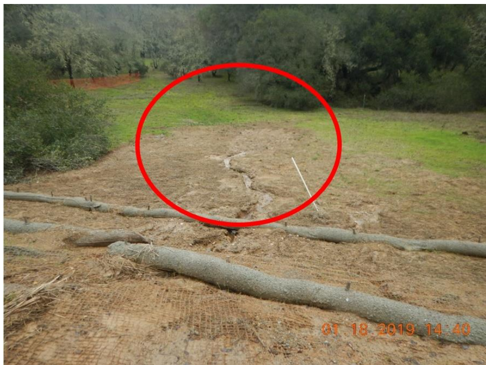
Figure 22. Sediment deposition beyond the undermined and overwhelmed BMPs; insufficient maintenance of erosion and sediment control BMPs.
