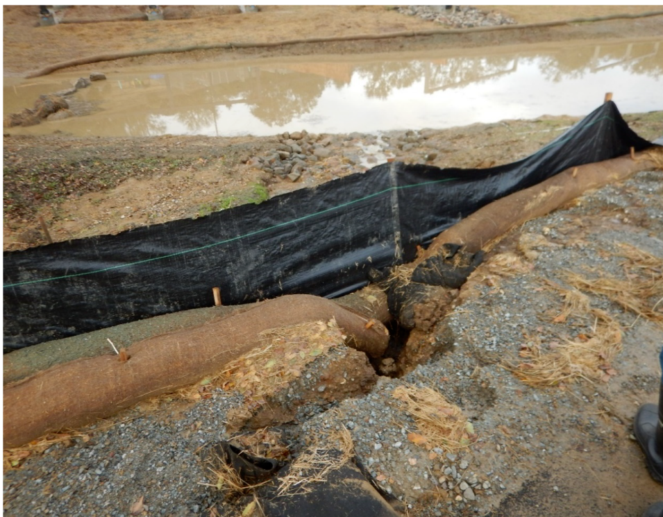
Figure 11. Erosional gully underneath wattle and silt fence; creek in the background.
