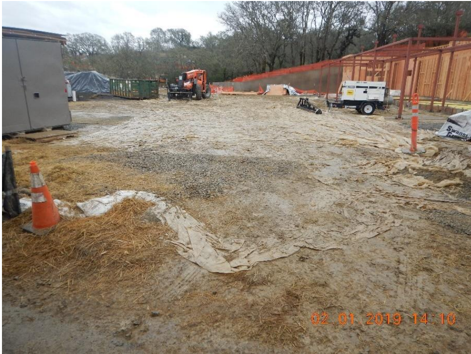
Figure 31. Ineffective erosion and lack of sediment controls in this inactive area.
