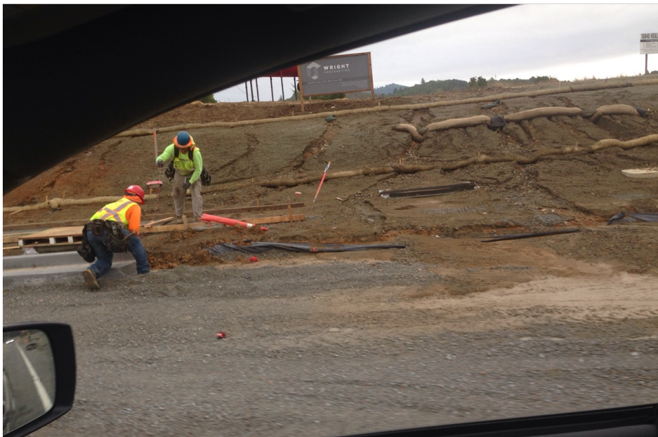
Figure 2. View of failed BMPs. Insufficient ground cover, and sediment in street (Healdsburg Avenue) after storm event. Photograph taken on October 3, 2018.
