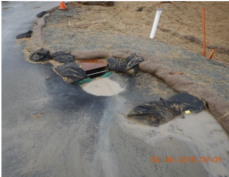
Figure 39. Sediment controls near the drainage inlet are not effectively reducing or preventing pollutants in storm water discharges.
