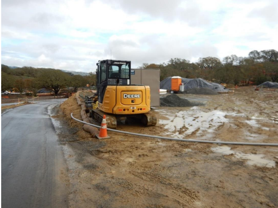
Figure 9. Disturbed soil where resort area was under active construction; lack of effective erosion or sediment control BMPs.
