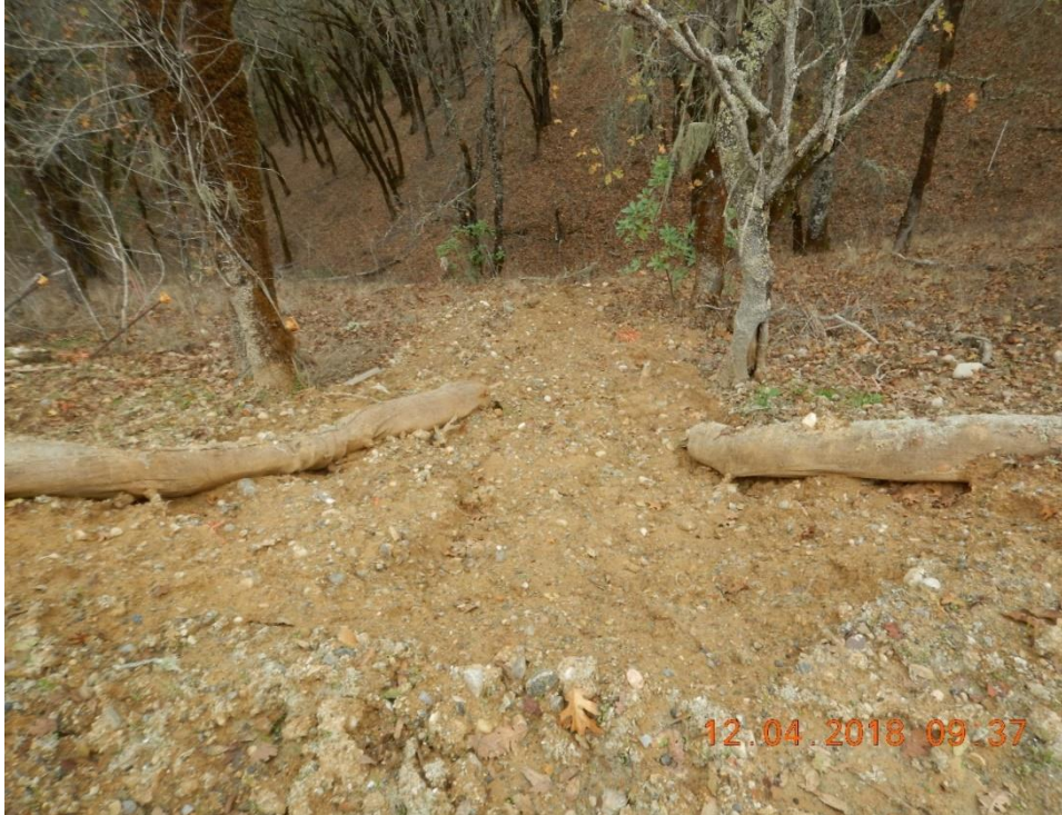
Figure 8. Sediment from Road 5 has breached the single perimeter wattle and discharged to the hillslope below. An unnamed tributary to Foss Creek is located approximately 75 feet downslope.
