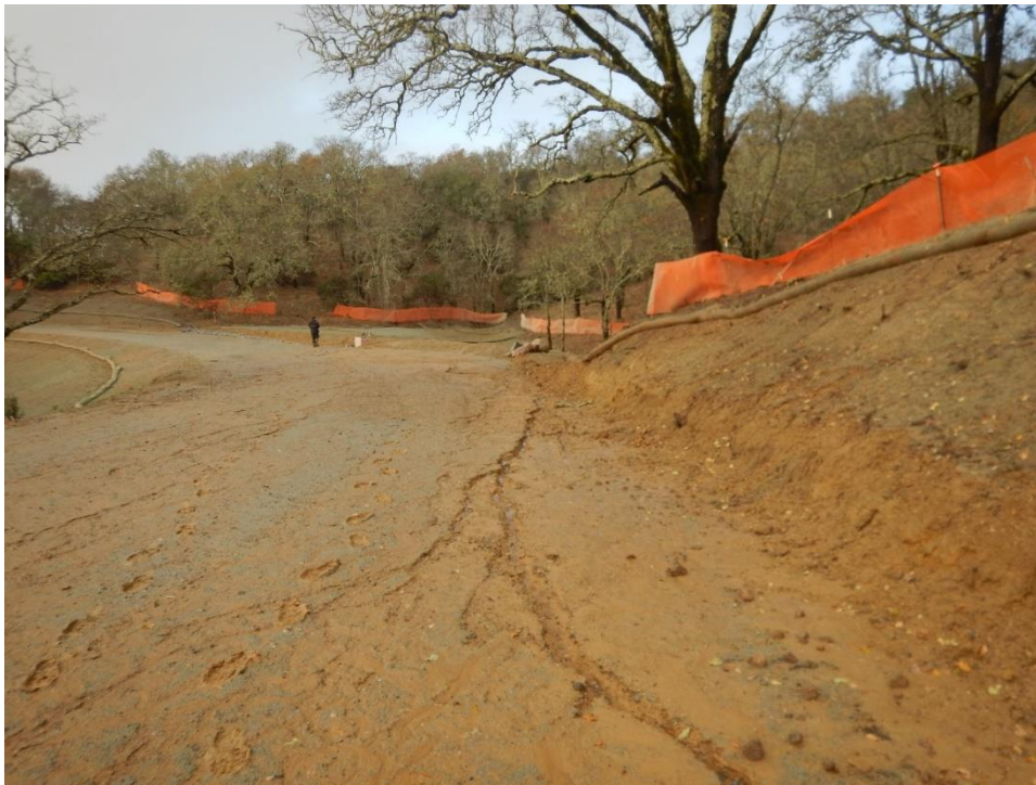
Figure 10. No linear sediment controls along the base of this roadside slope. Signs of gullying on the road.
