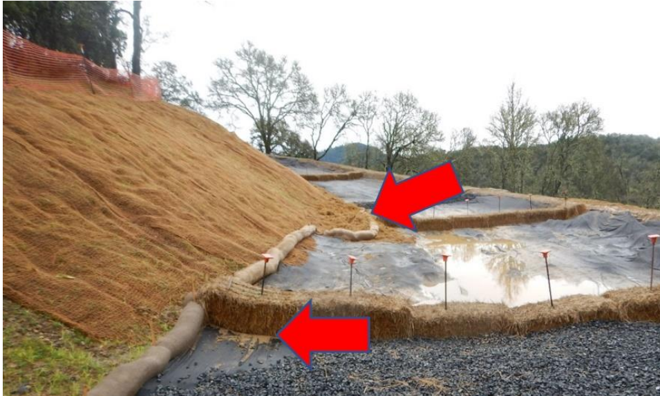
Figure 41. Note slumping slope on roadway. Turbid water is visible emerging from the left side of the first straw bale berm in the foreground. This turbid water eventually discharged to an unnamed tributary to Foss Creek.
