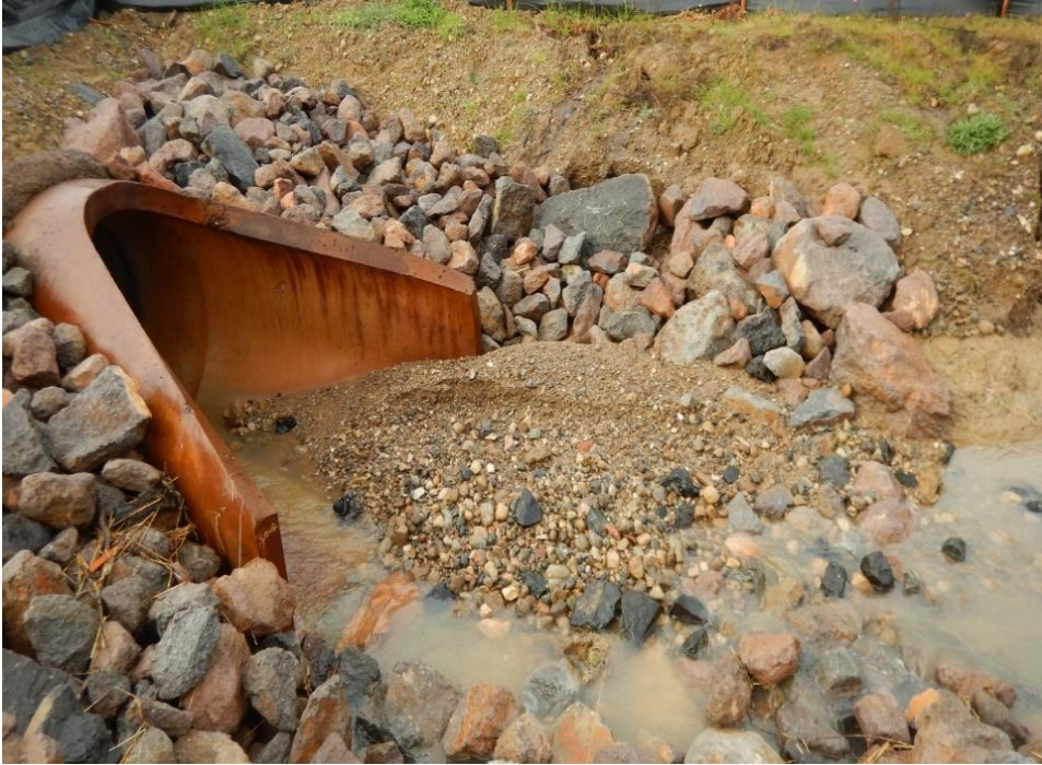
Figure 18. Downstream from Figure 14, large sediment deposit within Foss Creek as a result of the slope failure along the creek bank.
