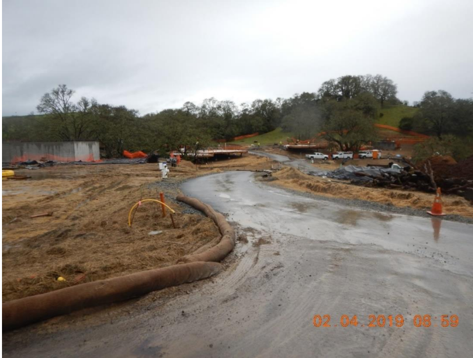
Figure 36. Poor maintenance of BMPs, and lack of BMPs to keep the paved roads clean continues to result in discharges of sediment-laden runoff to the drainage system.
