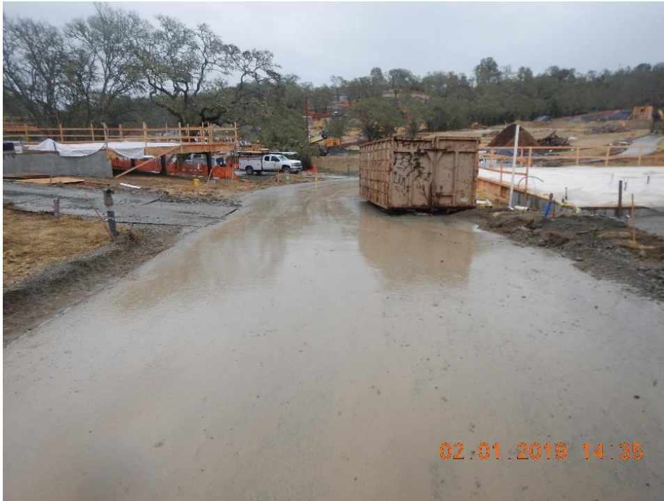
Figure 30. Mud on paved roads continues to result in discharges of sediment-laden runoff.
