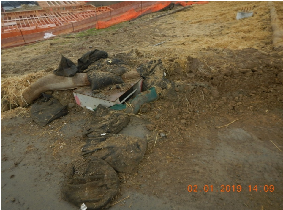
Figure 33. Sediment from the adjacent work area is overflowing onto the roadway and into the drain inlet.
