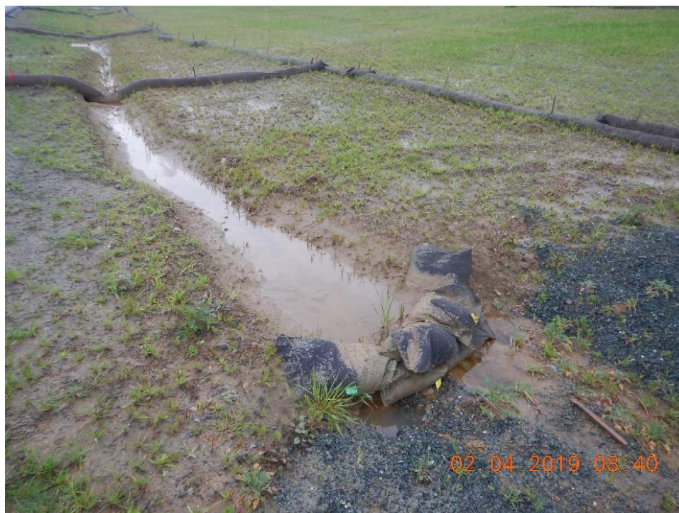
Figure 37. Erosion controls (hydroseed and straw soil cover) are not adequate or established enough to prevent sediment-laden runoff to the storm drain system that discharges to Foss Creek.
