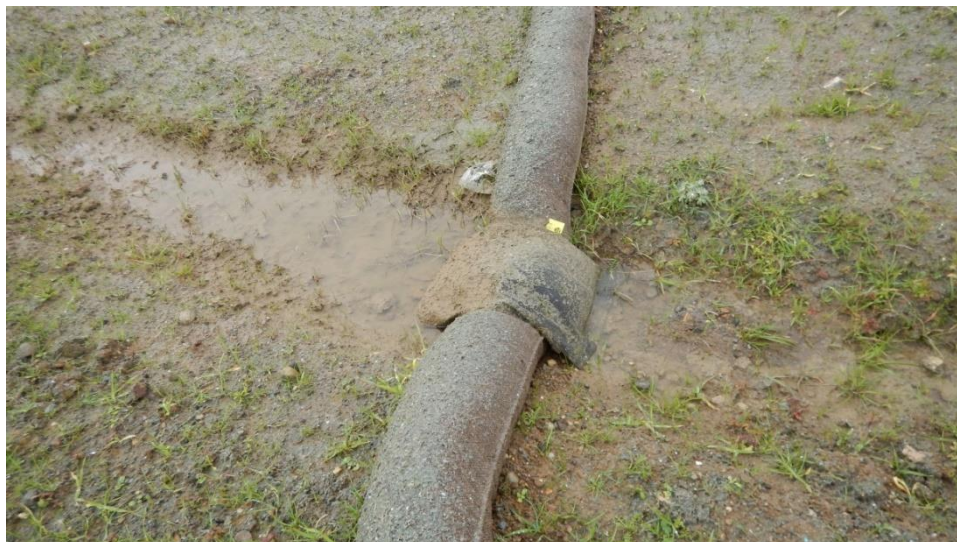
Figure 19. Ineffective soil cover contributing to erosion. The combination of BMPs for erosion, sediment, and turbidity controls on the Site was not adequate to prevent erosion and sedimentation.
