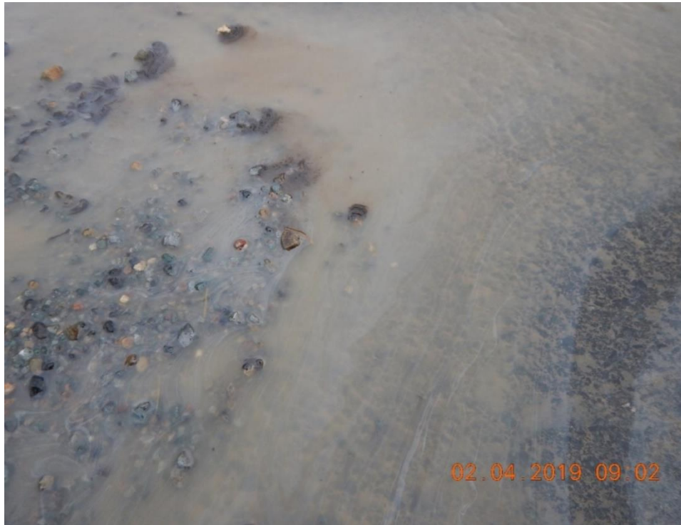
Figure 40. Oil sheen and turbid water on road surface in the resort area was observed flowing into the storm drain inlet in Figure 38.
