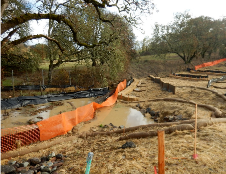
Figure 12. While several types of erosion and sediment controls are present at this location, the resort area lacked effective controls to prevent highly turbid runoff to the unnamed tributary (shown on left of photo) to Jordan Pond
