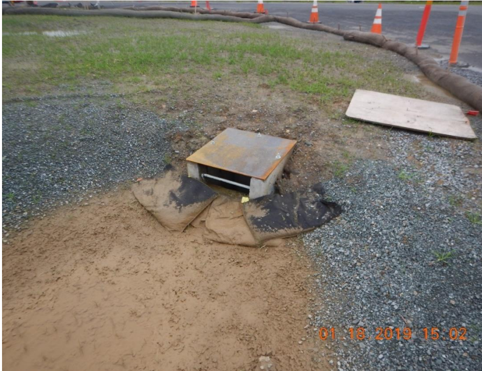
Figure 26. The sediment trap is inadequate and needs maintenance; sediment has overtopped the gravel bags and discharged sediment-laden runoff to the storm drain system that discharges to Foss Creek
