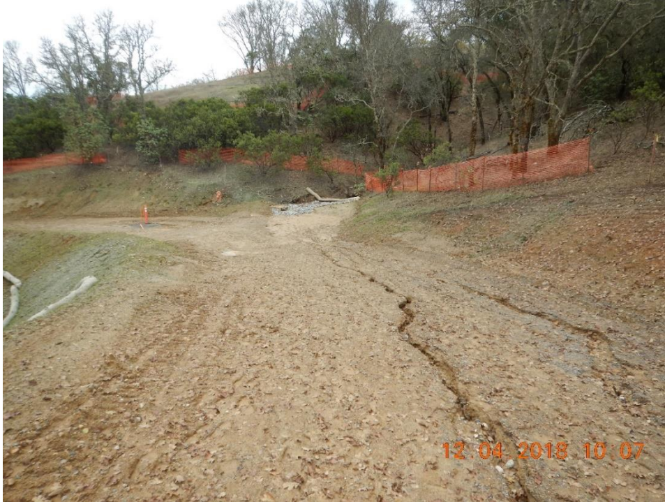
Figure 14. Road segment with no erosion and sediment control BMPs. Signs of gullying on the road.
