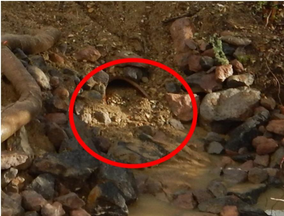
Figure 15. Significant sediment discharge at the culvert outfall that drains the upper resort area.
