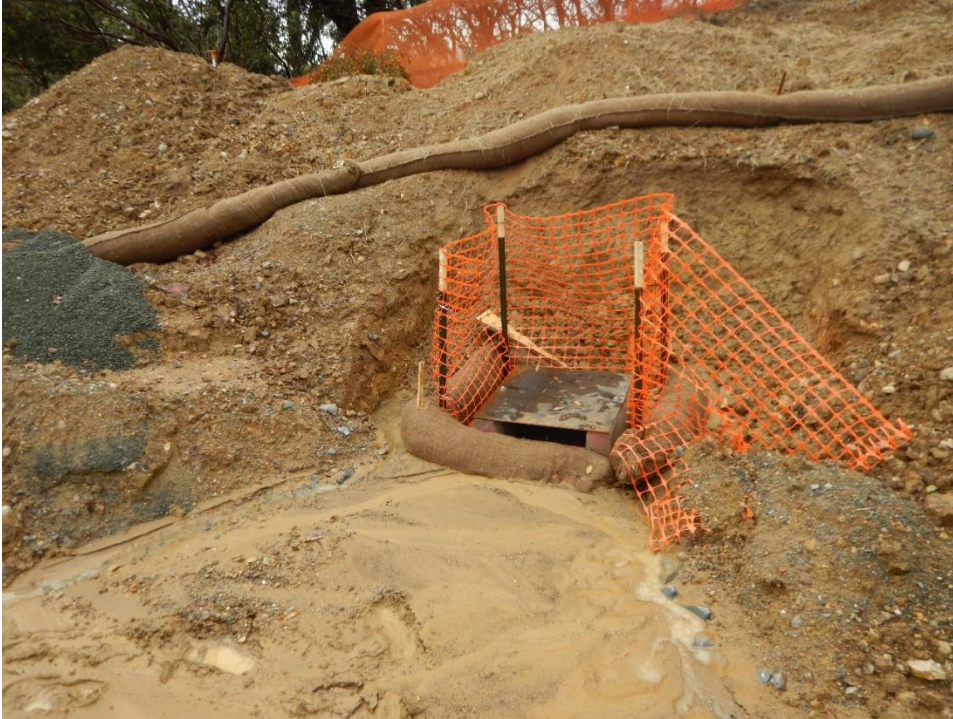
Figure 7. Sediment control BMPs inadequate to prevent erosion and overwhelmed by sediment deposition resulting from sediment-laden runoff.
