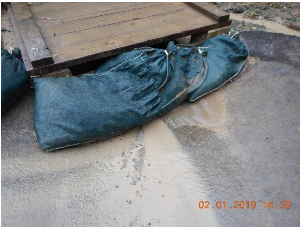
Figure 35. This check dam is not correctly positioned to effectively capture or remove pollutants from storm water runoff.
