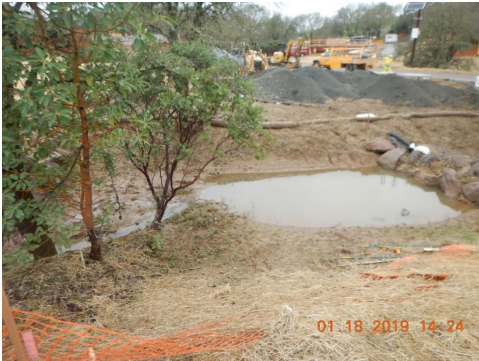
Figure 21. Uncovered stockpile near top of a stream/drainage channel bank. Creek in the foreground.
