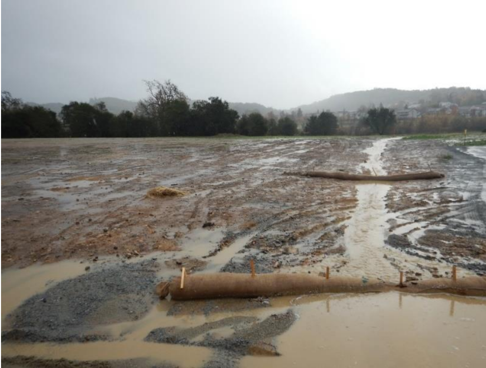
Figure 6. Ineffective Sediment control BMPs resulting in turbid, sediment-laden storm water runoff.
