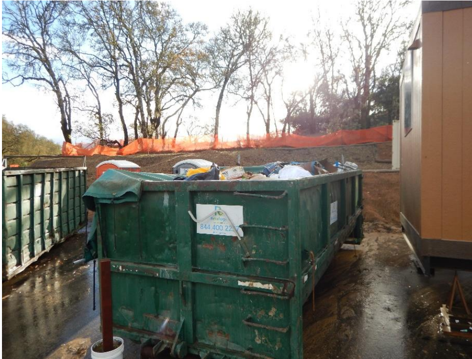
Figure 4. Uncovered waste disposal bin.
