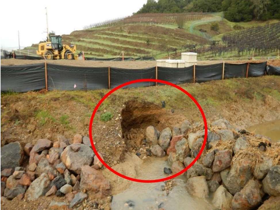
Figure 17. Lack of erosion and sediment controls in this inactive area resulted in stream bank failure that led to sediment deposition within Foss Creek
