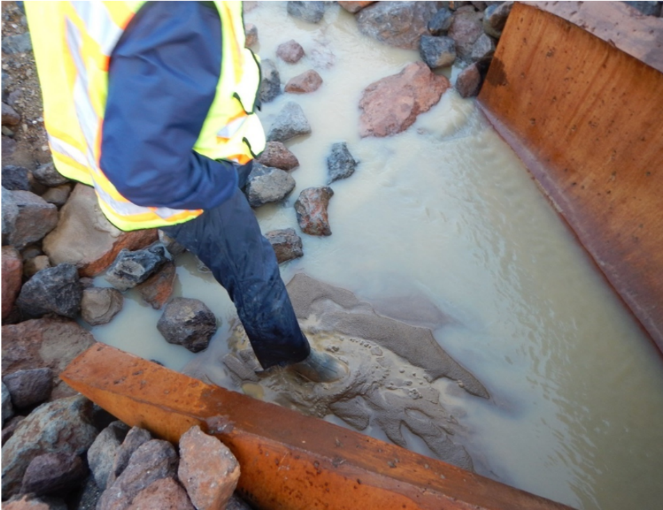
Figure 16. Significant sediment deposition within Foss Creek culvert inlet.
