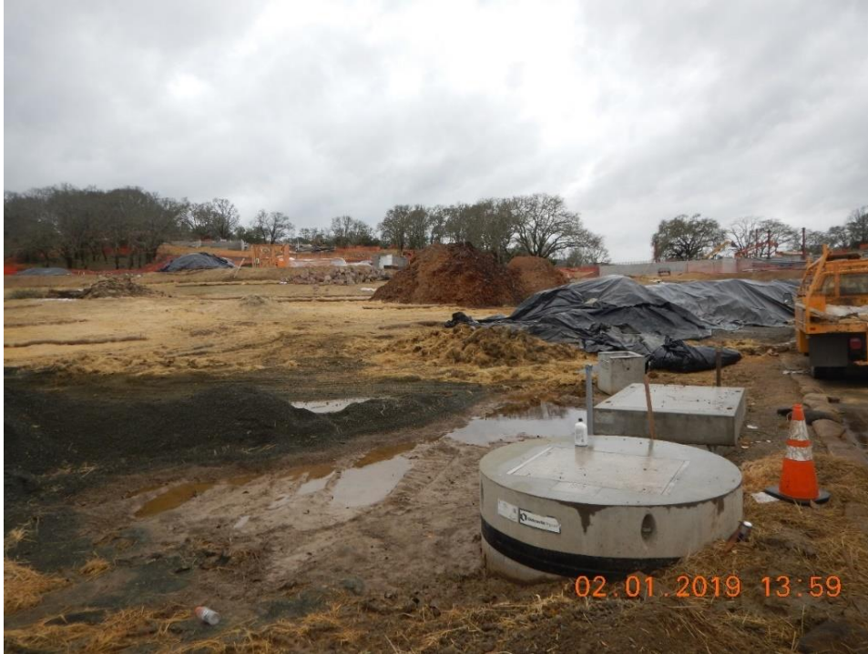
Figure 28. Stockpiles, some covered, some uncovered. Discolored water. Heavy equipment tracks in the mud.
