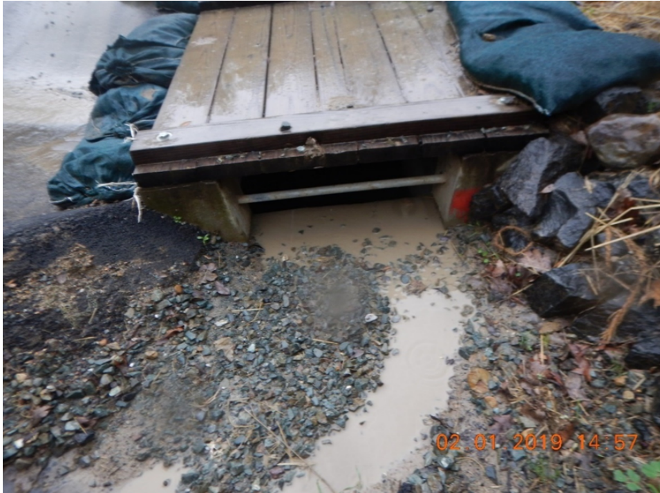
Figure 27. Turbid storm water runoff entering drain inlet that discharges to Foss Creek
