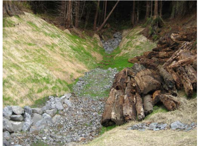
Figure 2. Stream crossing treated in summer 2007. Note rock armor in channel to minimize scour, logs and matting to minimize bank slumps over the extent of the excavation.
