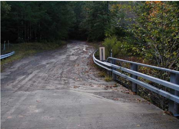
Figure 2 Road sediment draining to stream
