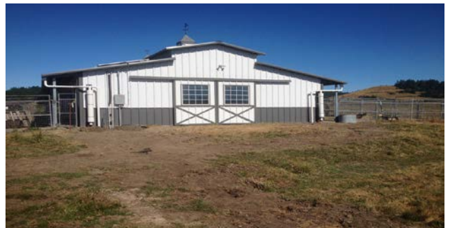
Photo 13: Downspouts from the 50,000-gallon tank collection roof and conveyance piping. The large diameter cylinders are the first flush diverters.
