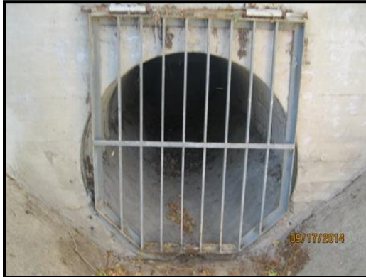
Figure 3: Outfall ID 44 with no flow.
