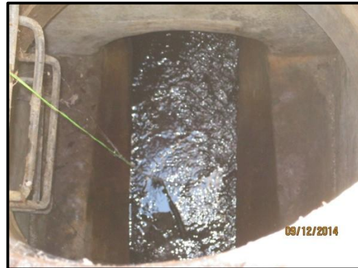
Figure 6: Outfall ID 100 with Substantial Flow.
