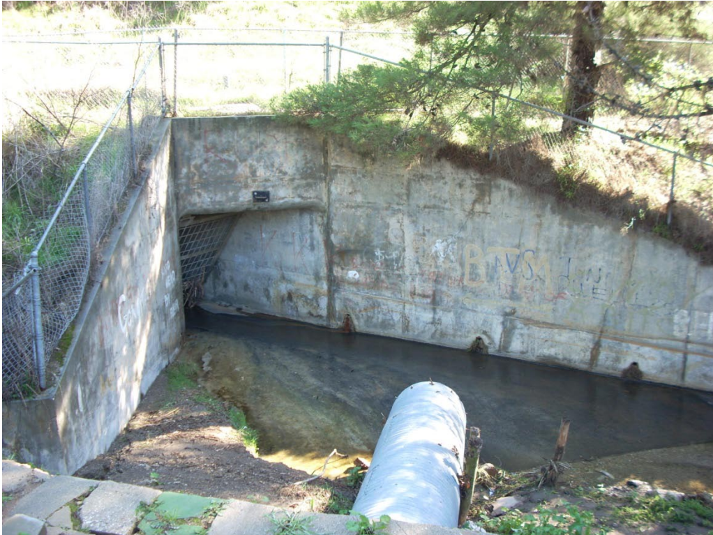
Figure 2.5 Valmonte Monitoring Site; Pipe Conveying Drainage from Valmonte Canyon is in the Foreground and Flow From Ferncreek Enters From the Right
