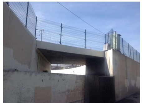
Discharge to Dominguez Channel
