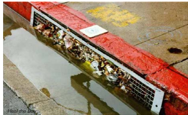
A clogged catch basin in Los Angeles.
