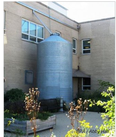
A large cistern collects roof runoff from a commercial building in Chicago.
