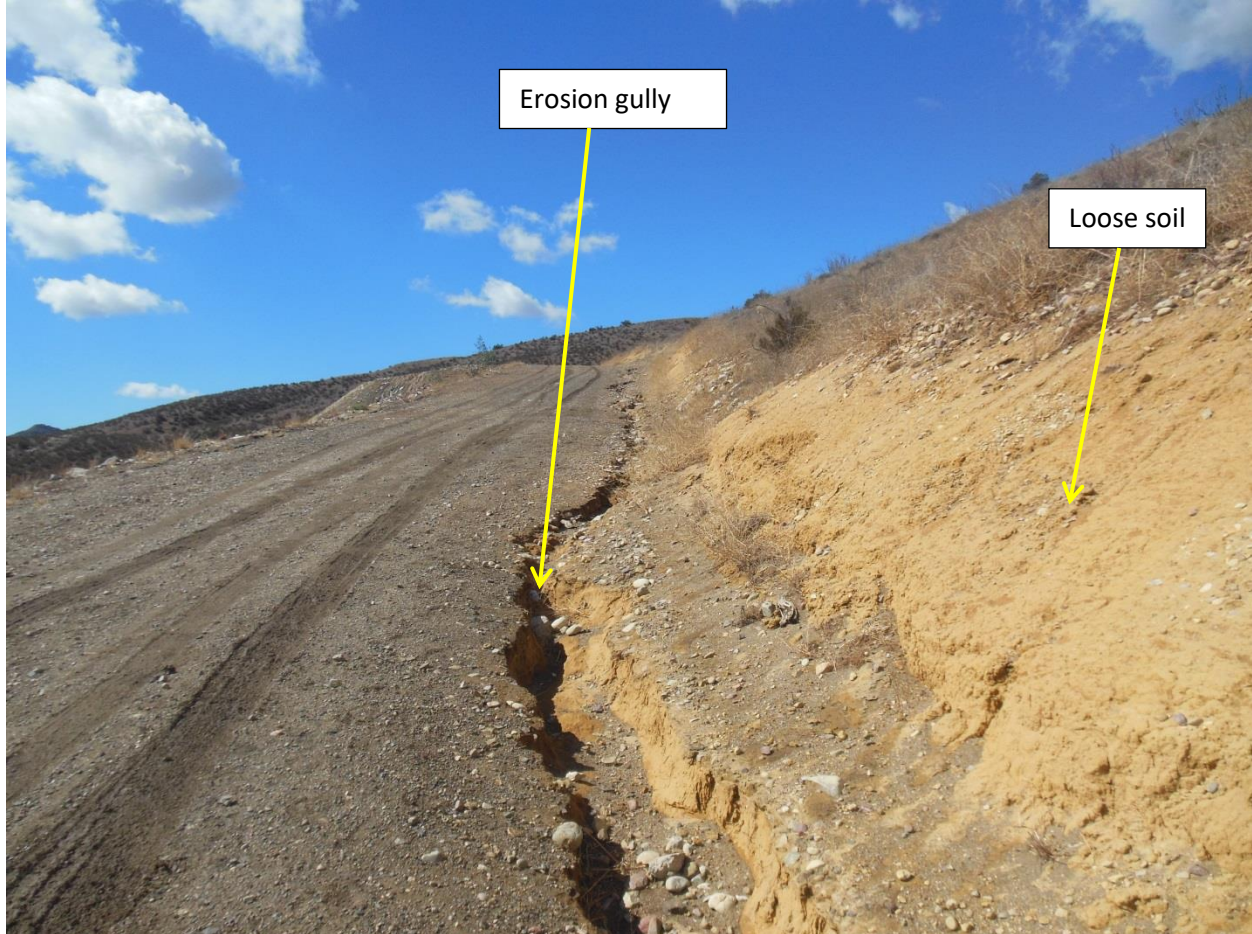
Photo 25. This photo shows a dirt road with an erosion gully running along its edge. This photo was taken in Parcel 2821-009-030 near latitude: 34 18.260 and longitude: -118 36.831. This area lacked erosion control BMPs.
