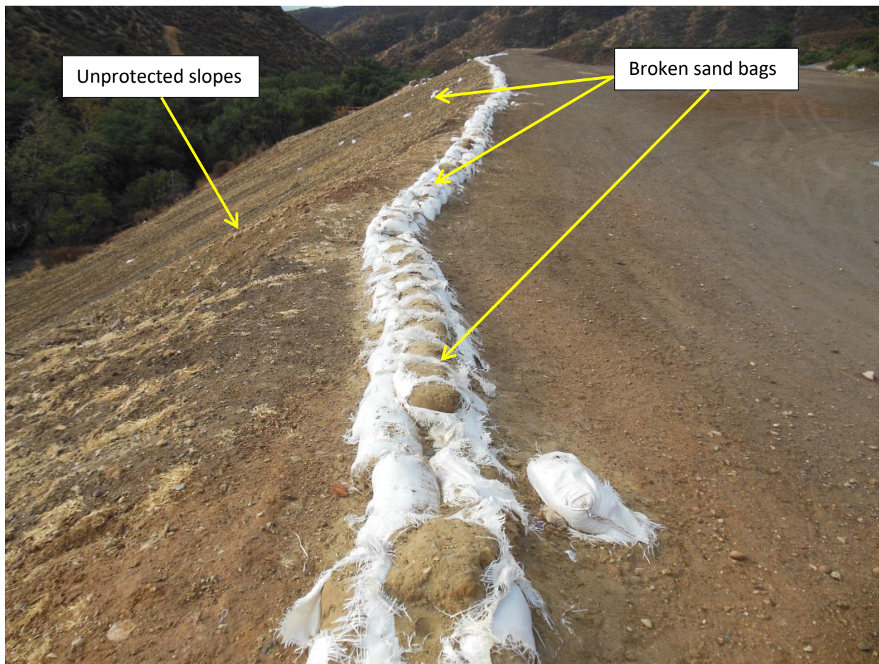
Photo 27. This photo shows a damaged sand bag berm placed at top of slope at the edge of an area that was graded flat. This photo was taken in Parcel 2821-009-031 near latitude: 34 18.264 and longitude: -118 36.644.
