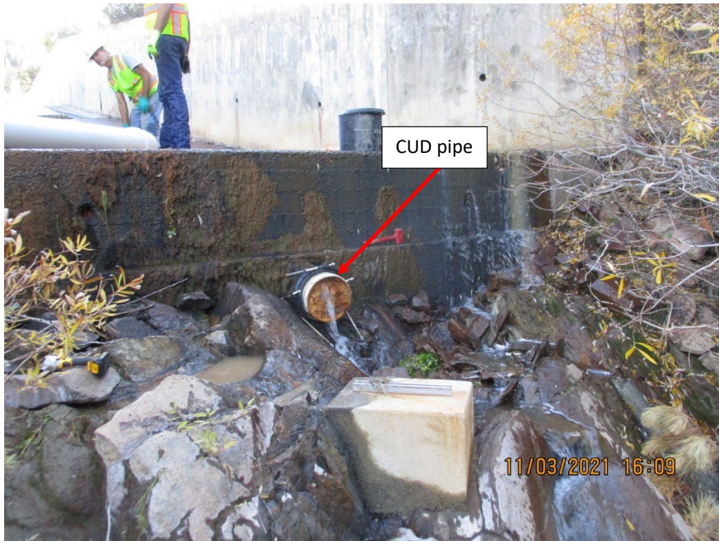
Photo 7 – November 3, 2021, Metal precipitates at the downstream end of the CUD pipe
