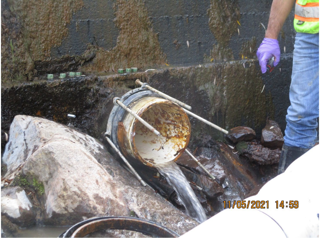
Photo 11 – November 5, 2021, CUD pipe after removal of metal precipitates (prior to reinstallation of the outlet pipe to weir box)
