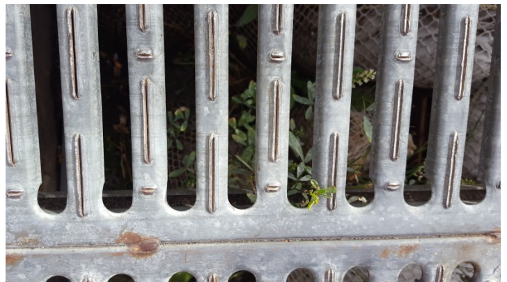
Photo No. 2 Sierra Boat Company: Hydrographic Area A, weeds growing out of stormwater inlet.
