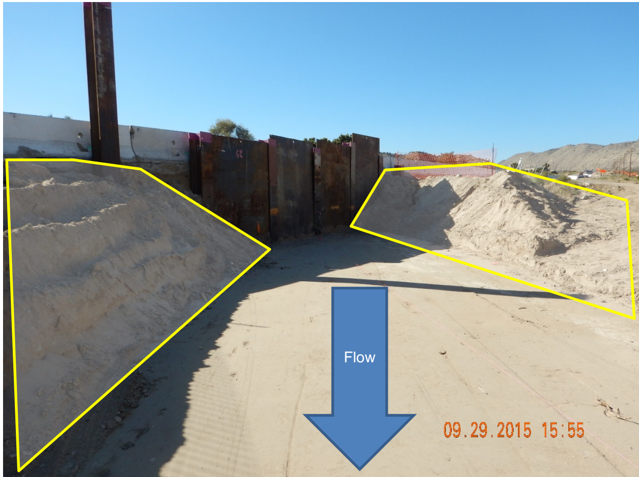
Picture 9: View West at Drainage ID 16. Note the un-stabilized stream banks and absence of erosion and sediment controls (approximate areas in yellow boxes). Additionally the stream has been completely disconnected from upstream flow with metal sheet pilings.
