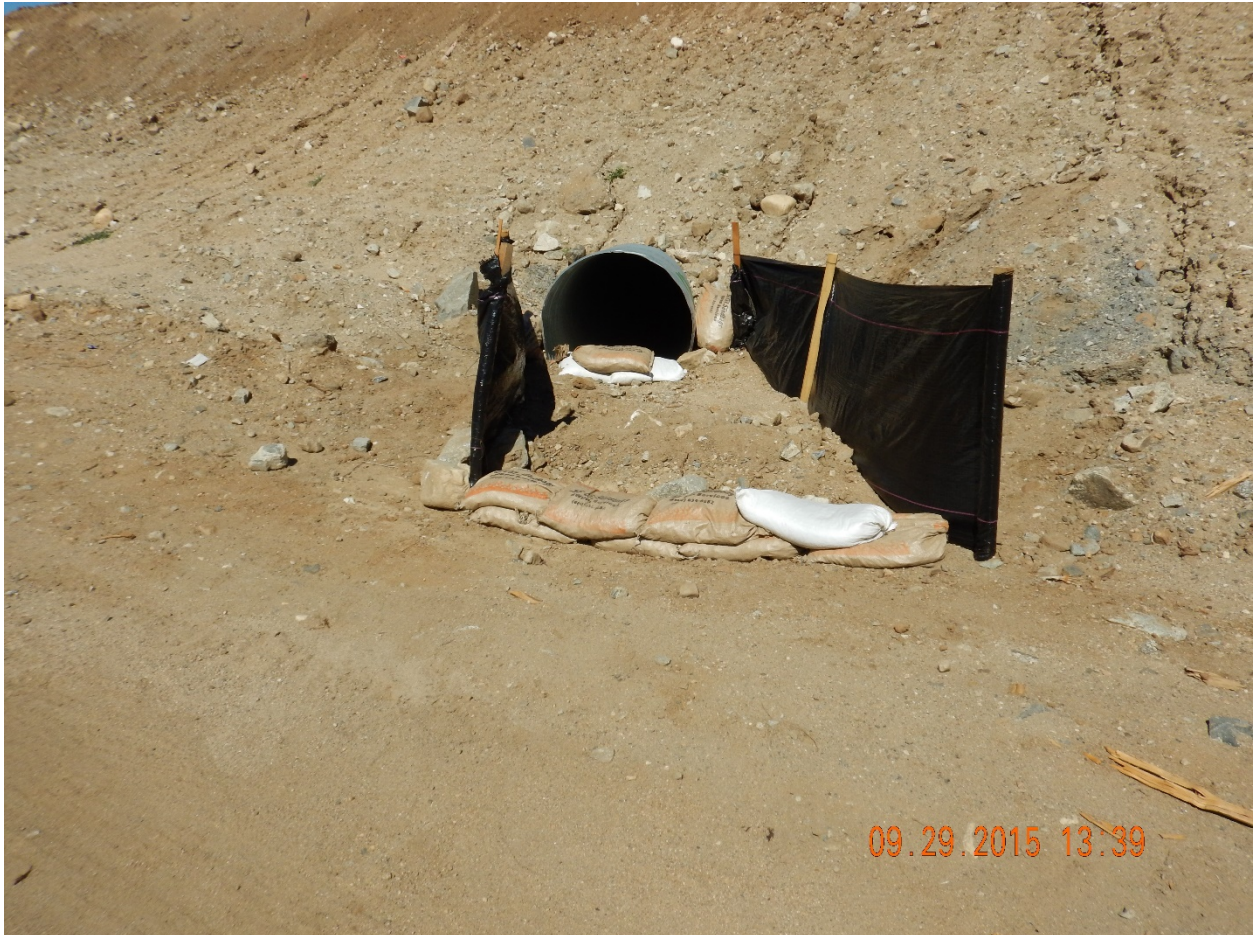
Picture 7: View North of Drainage ID 55. Note the inadequate BMPs and unconsolidated sediment and sandbags in the stream channel.
