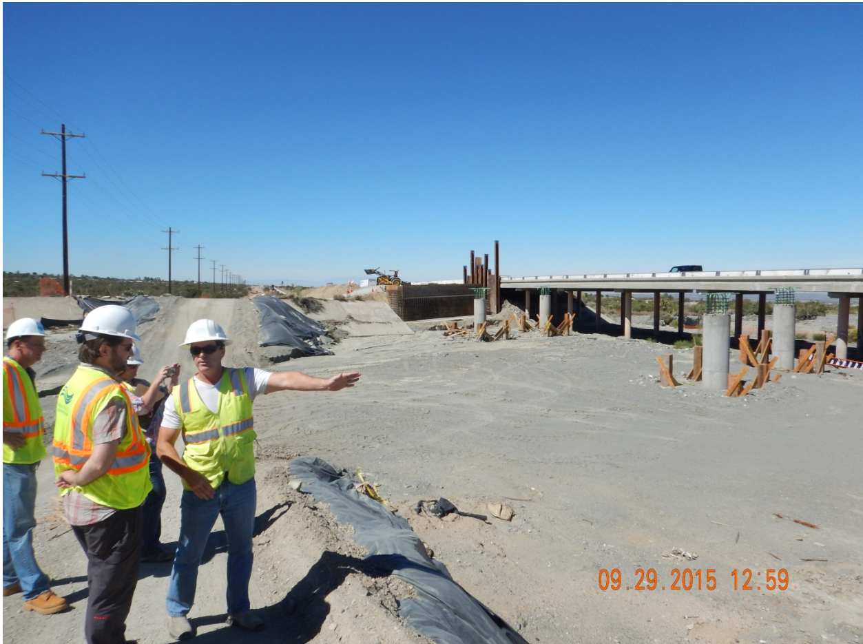
Picture 24: View North West from eastern bank of Sheep Creek. Note Construction Access Road through the Creek with inadequate BMPs.
