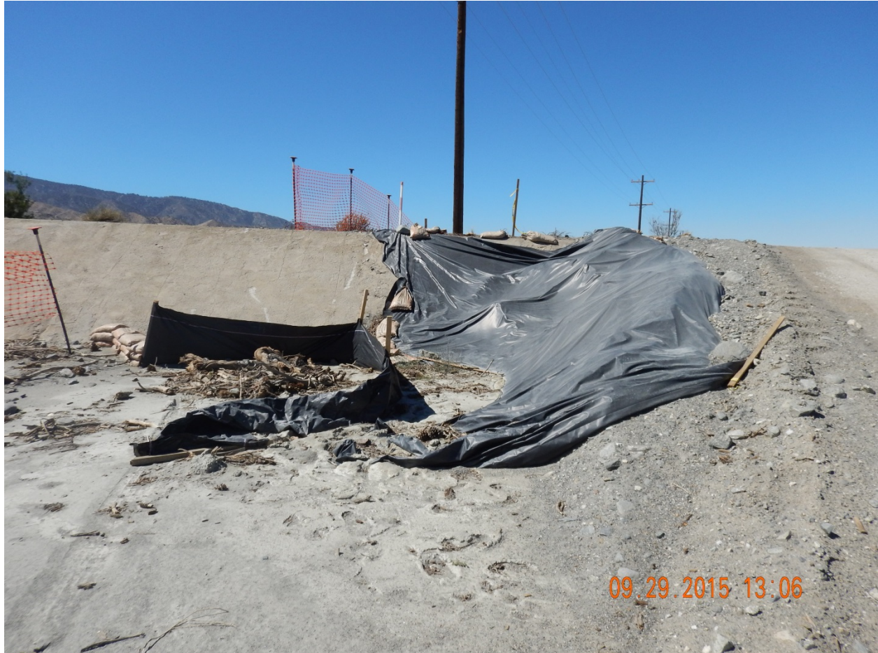
Picture 28: View West from within Sheep Creek. Note inadequate BMPs and failing improperly installed silt fencing.
