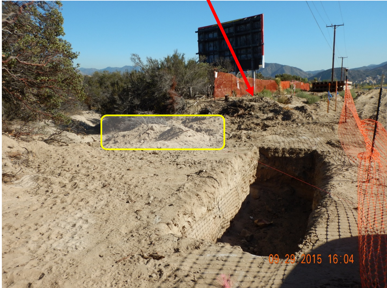
Picture 8: View South East of Drainage ID 69. Note excavation in channel, spoils from excavation stockpiled adjacent to excavation and in channel (shown in yellow rectangle), and no erosion and sediment controls installed.
