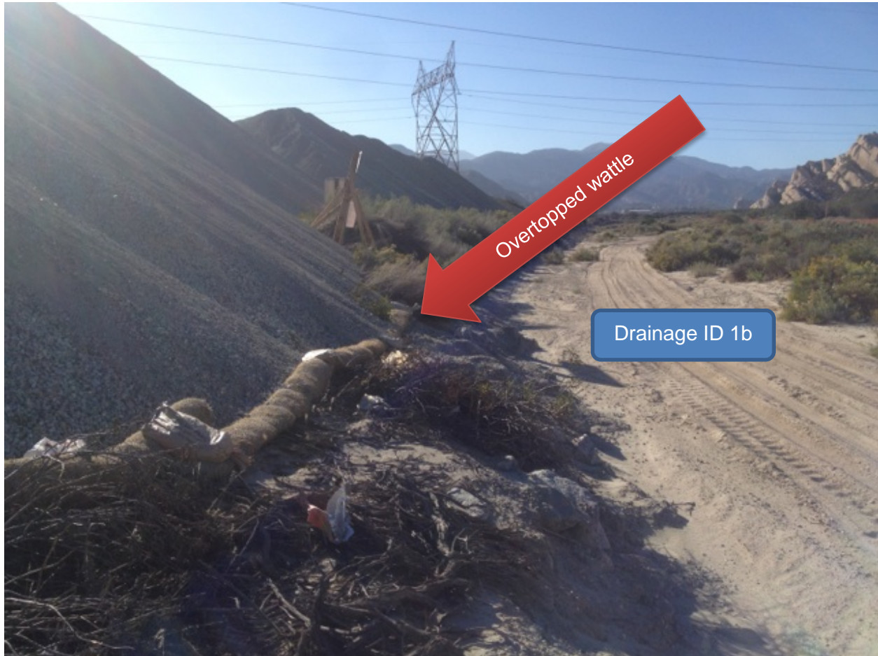
Picture 11: View North West of Drainage ID 1b. Note the large stockpile of gravel adjacent to water body and overtopped wattle with gravel in streambed.
