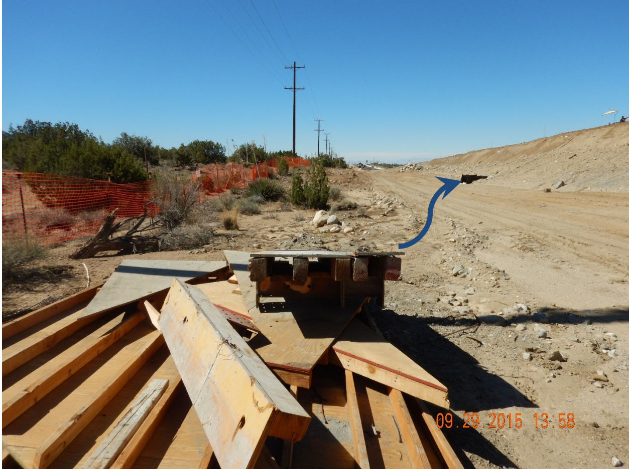
Picture 6: View West of unpermitted temporary impact at Drainage ID 55. Note the access road parallel to road construction and fill within the stream channel. Flow path and direction shown with arrow.
