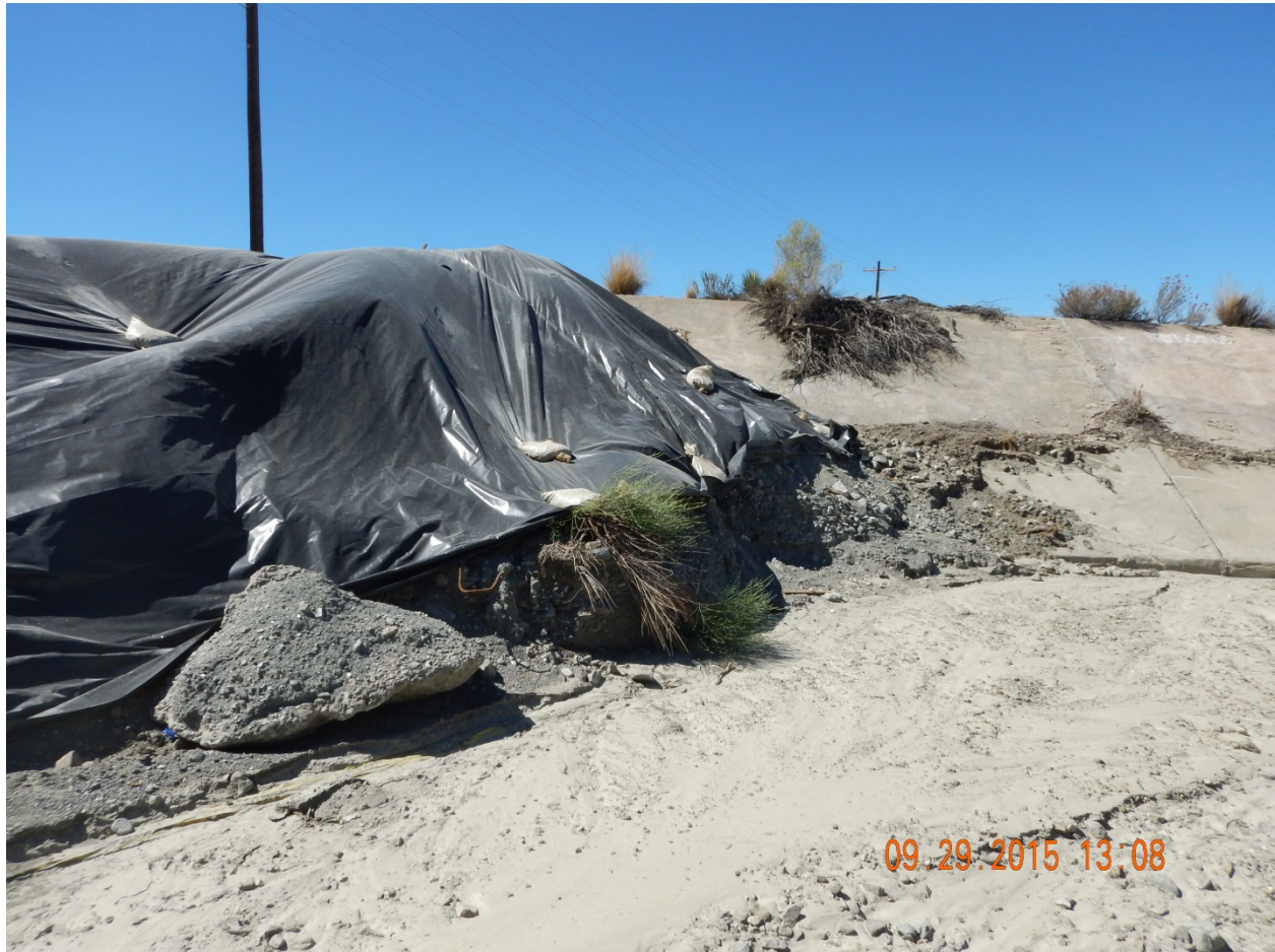
Picture 27: View West from within Sheep Creek. Note inadequate BMPs.
