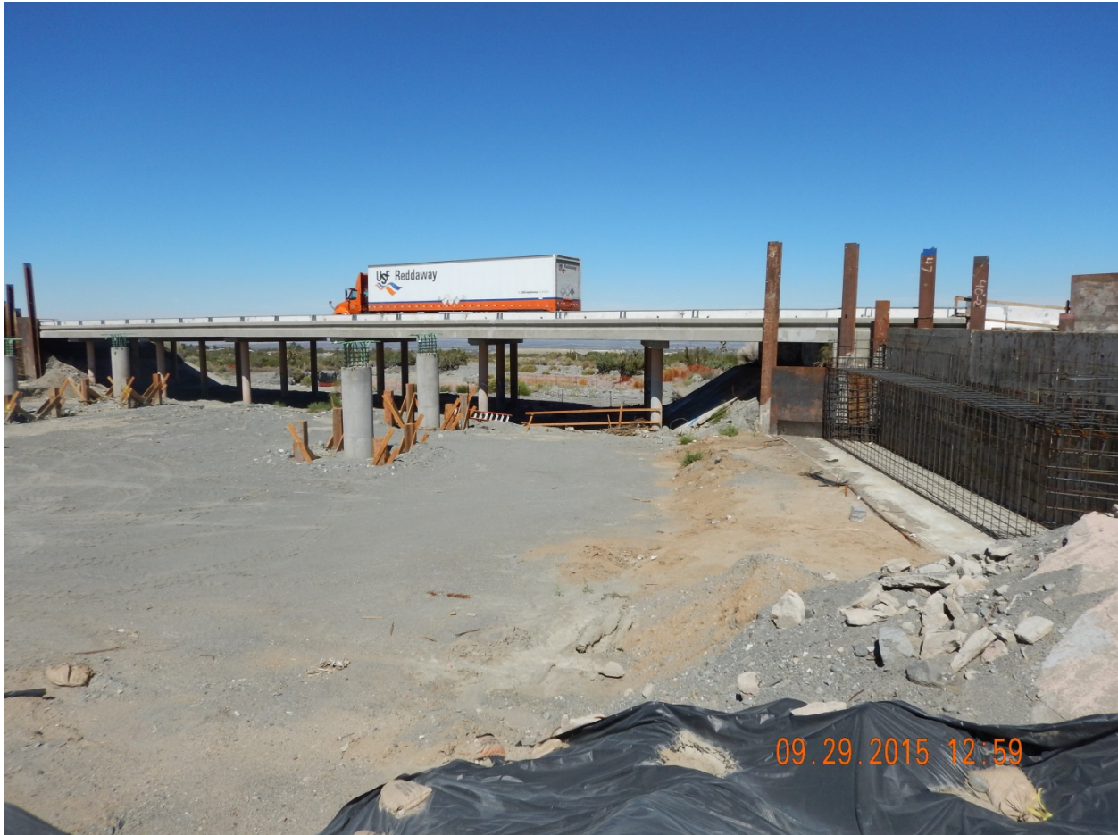
Picture 19: View North Within Sheep Creek. Note Extensive in-channel work and inadequate BMPs.
