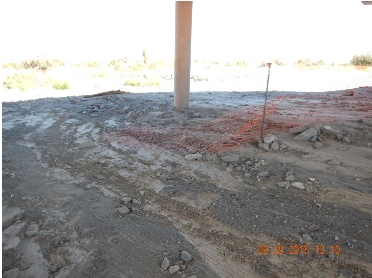
Picture 22: Beneath the Sheep Creek Bridge. Note damaged construction fencing left in the creek.
