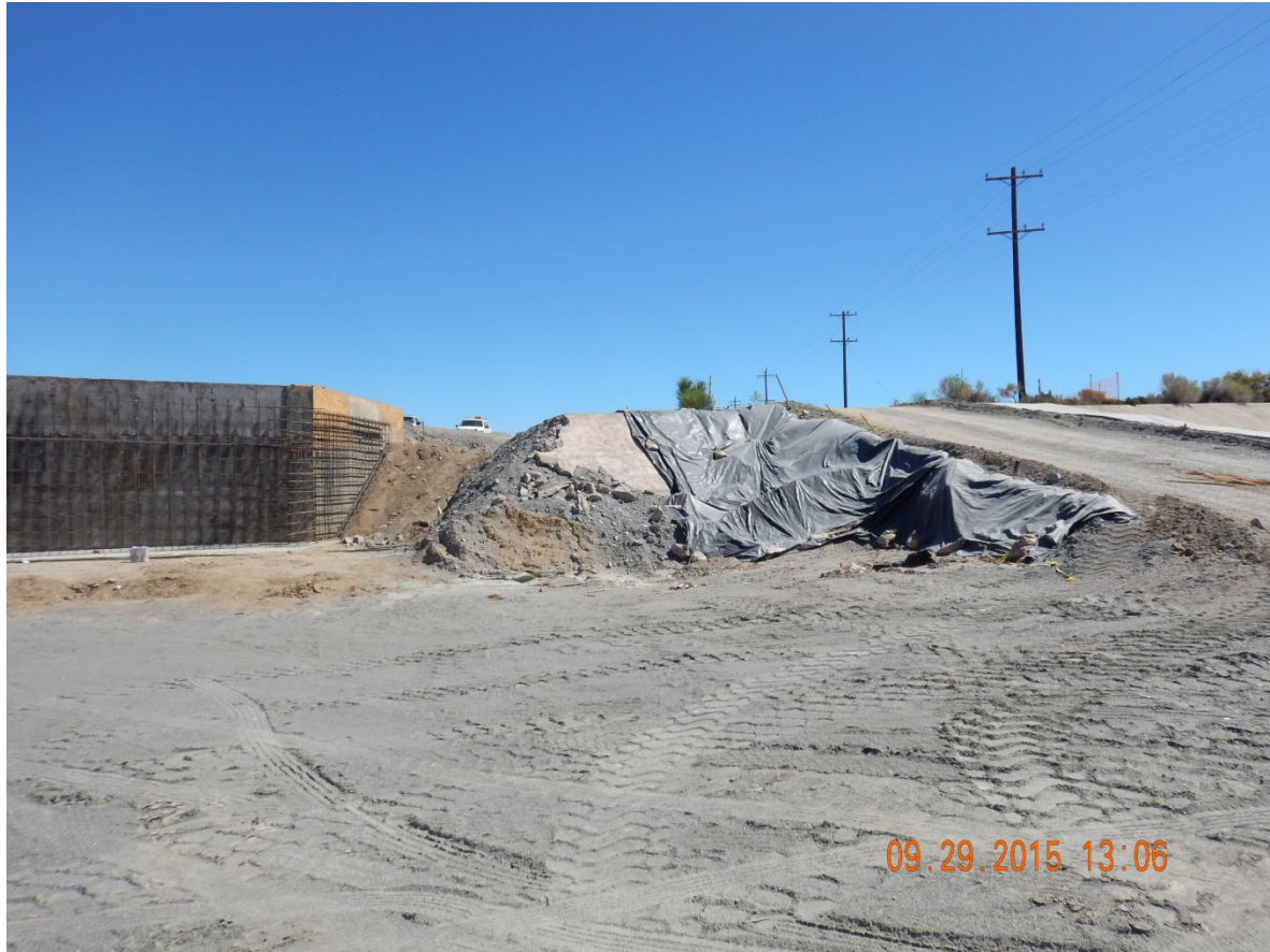
Picture 17: View to the East, From Within Sheep Creek. Note the lack of BMPs and failing BMPs.
