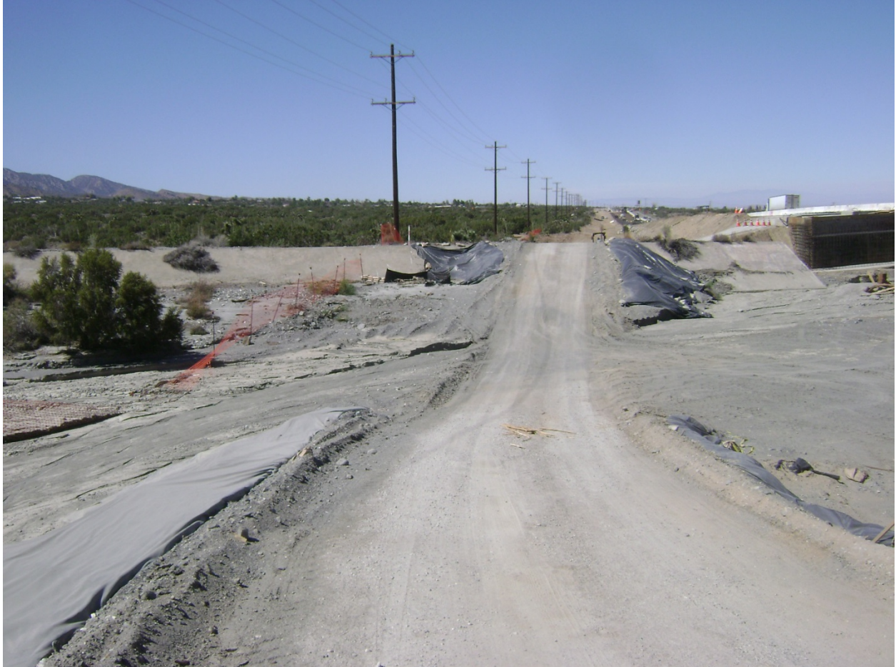
Picture 18: View to the West, From East Bank of Sheep Creek. Note Construction Access Road Crossing Through Creek With Inadequate BMPs.
