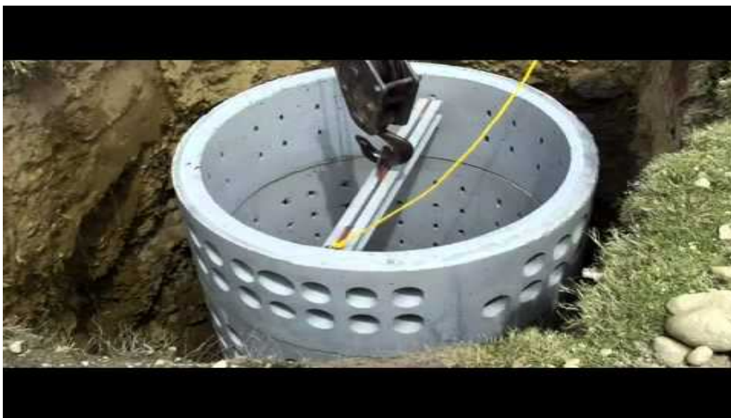
Figure 2 – The photo shows a seepage pit commonly used in the high desert. Instead of a Leach Field, effluent flows into a sub-surface pit and seeps into the surrounding soil.
