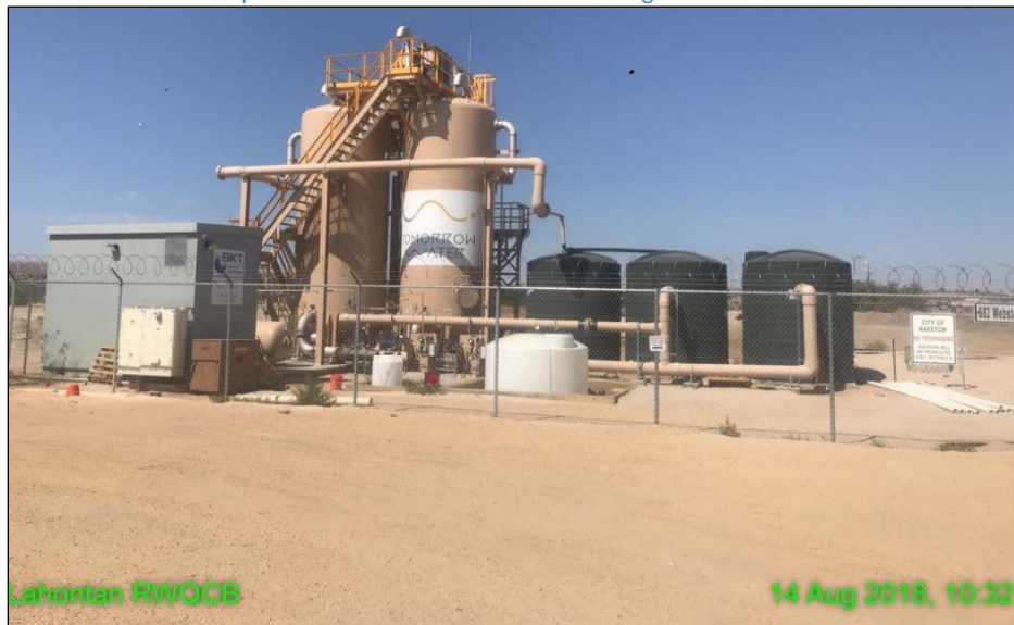
Figure 1 - BKT Pilot Project treatment vessels in the Soapmine Road area that is being tested for nitrate and perchlorate treatment of extracted groundwater.
