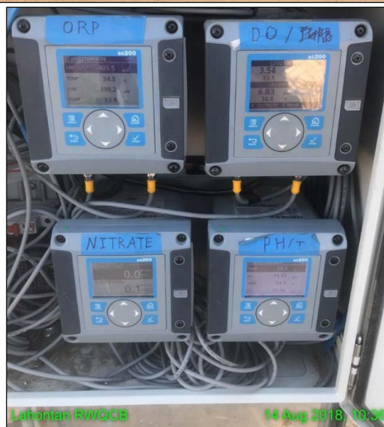
Figure 2 – Continuous measuring devices on the BKT pilot project equipment panel for testing of ORP, DO, NO 3 , and pH.
