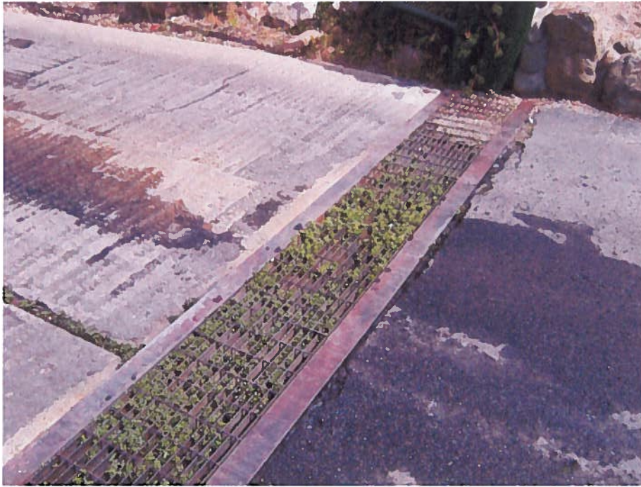
Photo 13. Clogged slotted drain along boat ramp, located on northeast side of the marina. Looking toward the east side of the ramp.
