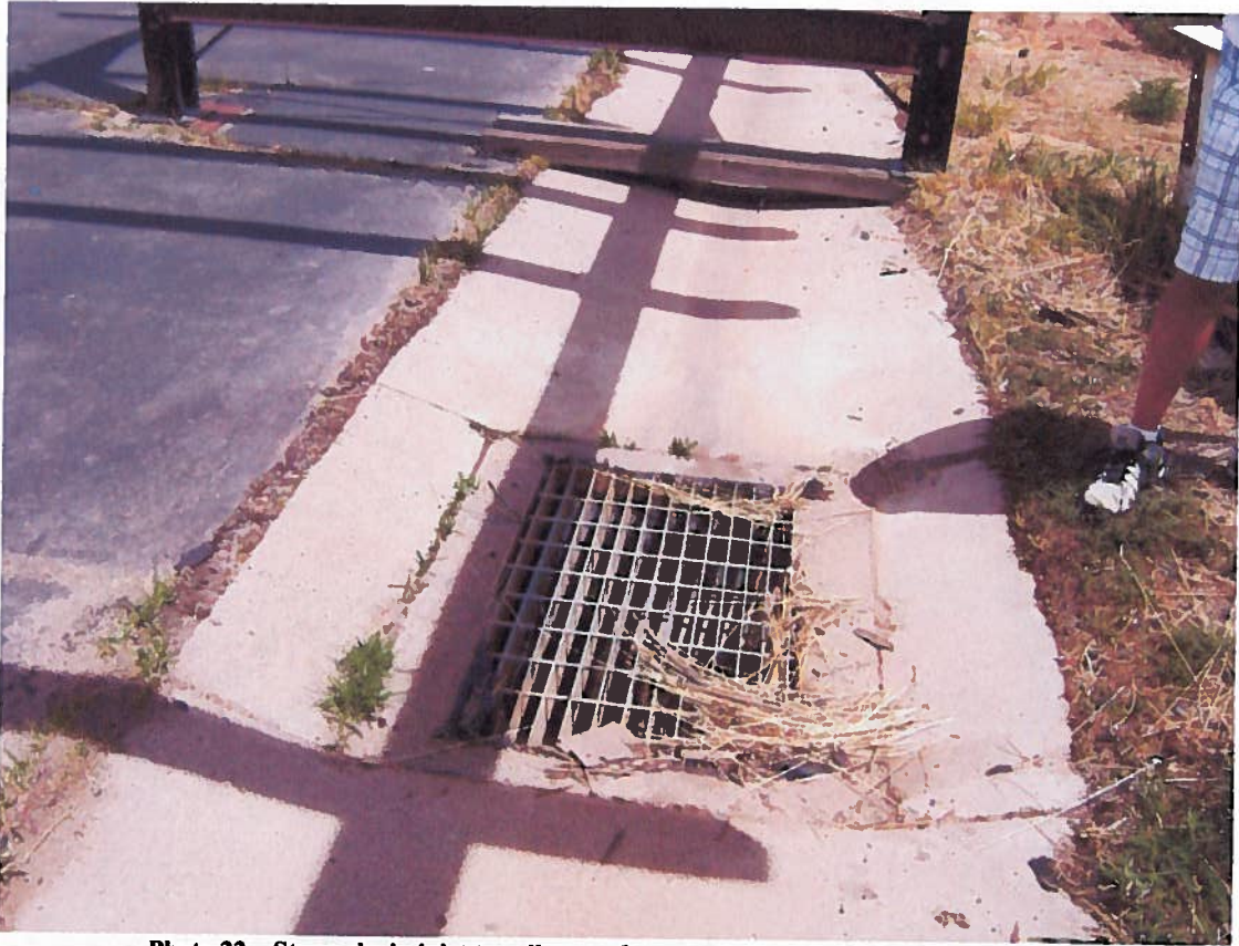
Photo 22. Storm drain inlet to collect surface runoff from boat storage area. Facing east.
