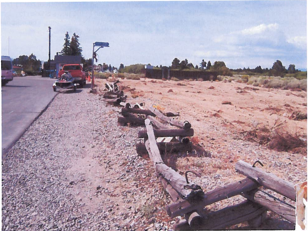
Photo No. 1. Looking northeast at graded area. Marina parking and boat ramp is on left. Existing graveled area abuts border between fenced area and parking lot.
