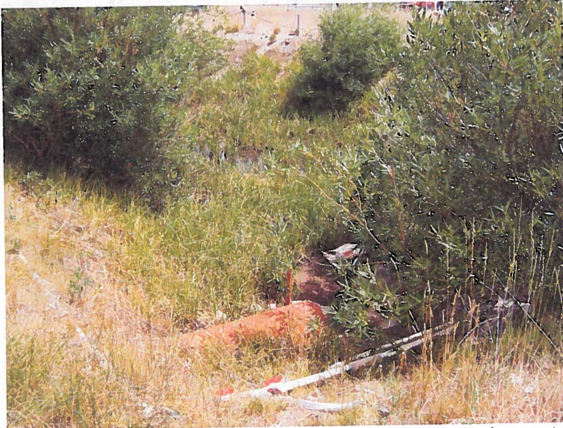
Photo 24. Discharge pipe (rust colored pipe in foreground) from stormwater treatment vault into the stormwater pond. Facing southeast.
