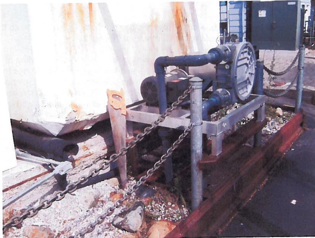
Photo No. 6. Sewage Pump-Out, located on northwest side of Fresh Ketch restaurant. Repairs had been made to facility earlier in the day, per Robert Spinnato.
