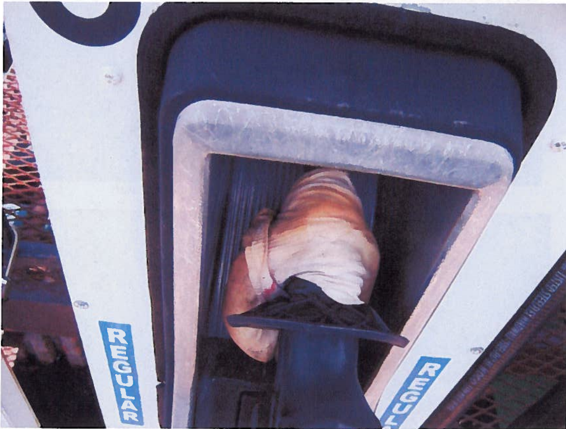
Photo 4. Gasoline-soaked absorbent material around pump dispenser.
