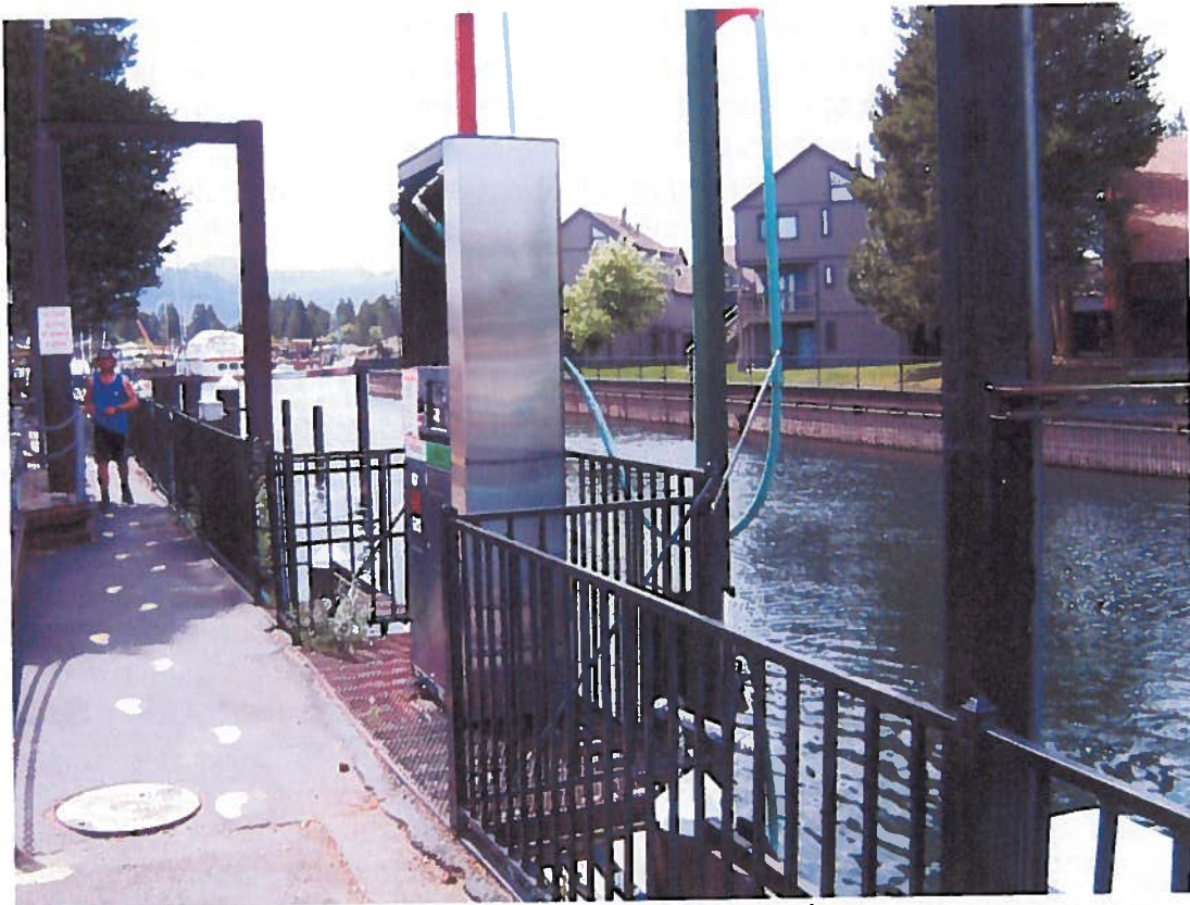
Photo 2. Diesel Pump, looking southwest.
