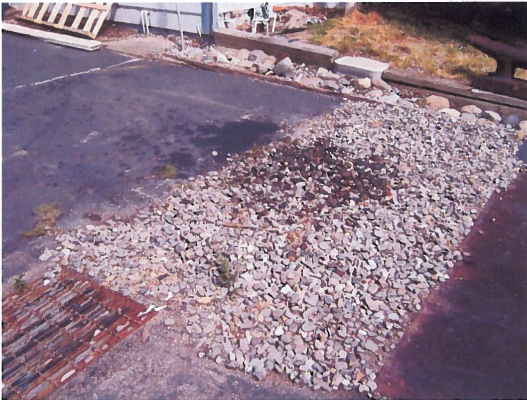
Photo No. 8. Antifreeze-stained gravel in drain rock on northwest corner of maintenance building. Looking southeast, marina bulkhead is immediately to the right of photo
