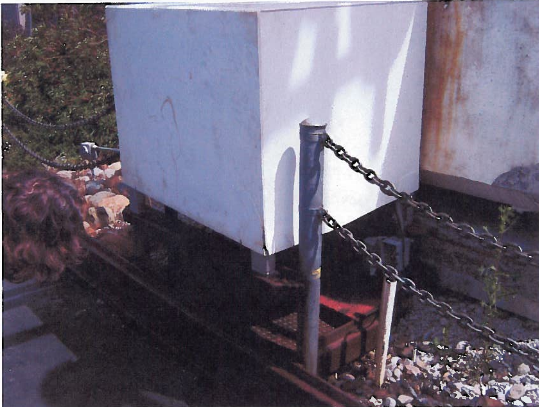
Photo 6. Sewage Pump Out facility, looking northeast. Silicon lubricant has spilled on rocks/rack below from ongoing maintenance activities to get it operational again.
