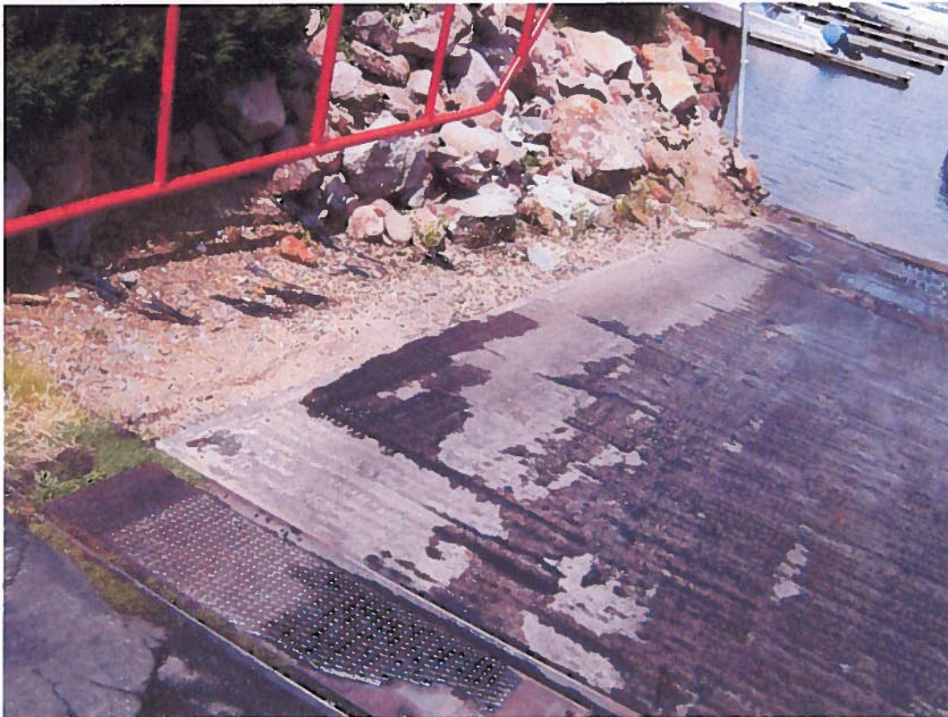
Photo 12. Clogged slotted drain along boat ramp, located on northeast side of the marina, along the west side of the ramp.
