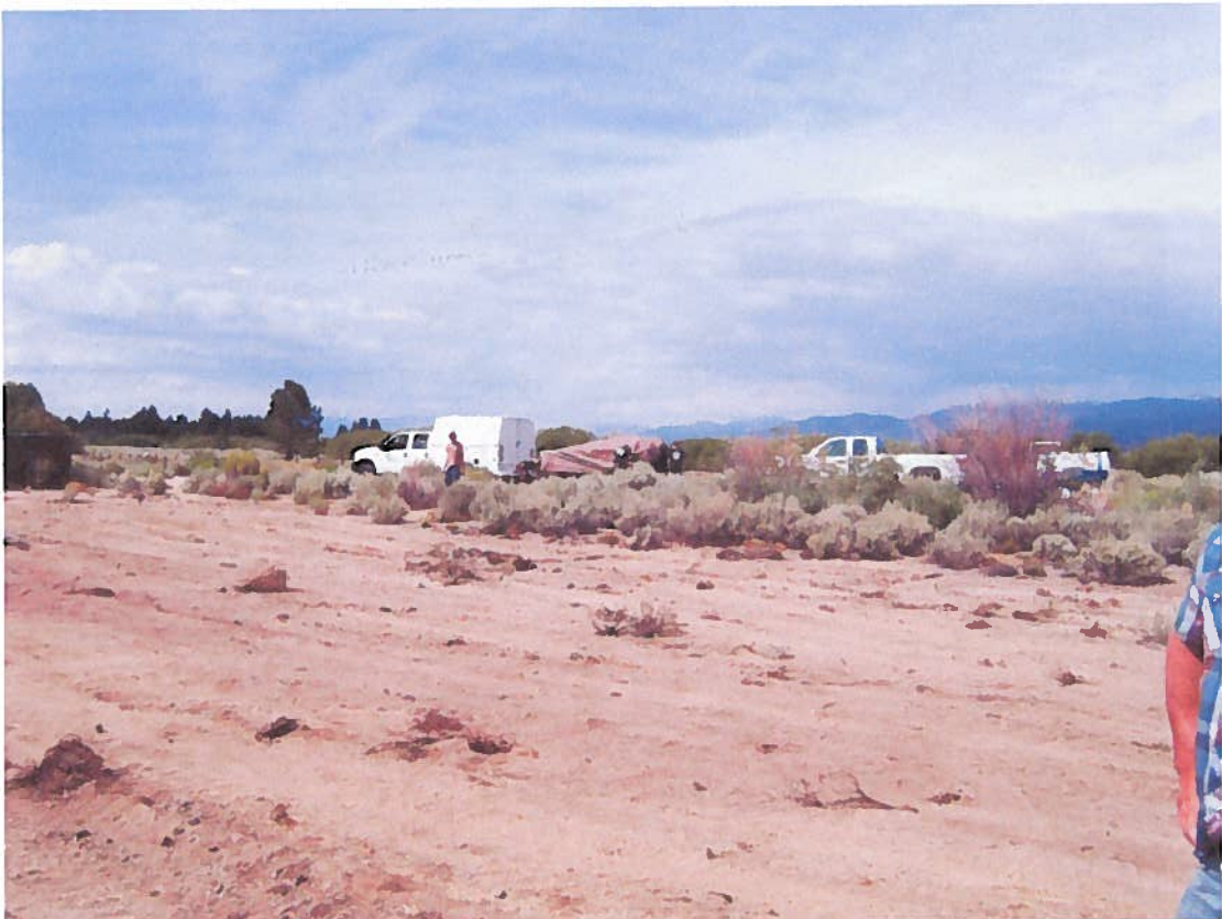
Photo No. 5. Looking east northeast at graded area, CTC crews arriving to install BMPs.
