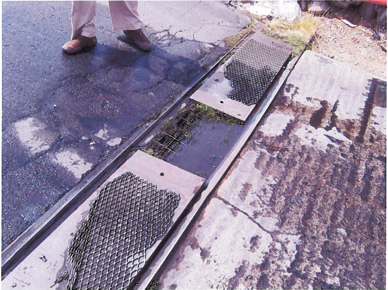
Photo 10. Clogged slotted drain along boat ramp, located on northeast side of the marina, looking toward the west side of the ramp.
