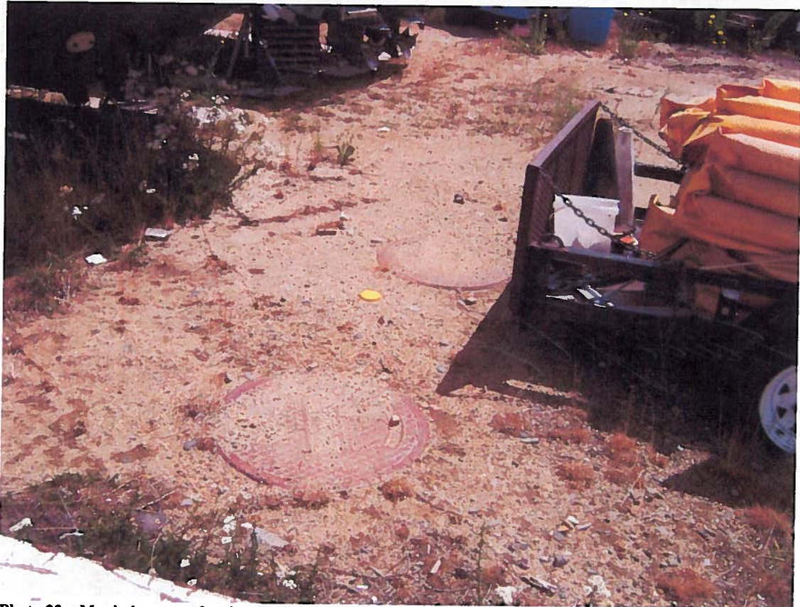
Photo 23. Manhole covers for the stormwater treatment system vault, located south to the drain inlet. Facing south.
