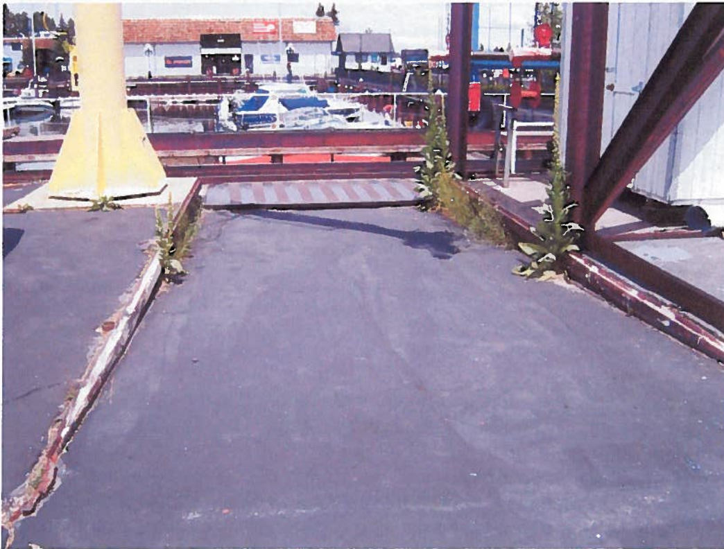
Photo 20. Ramp area on southwest side of boat lift, facing northeast toward maintenance building. (Fishing Charter business is in the small building to the right of the maintenance building, and the drain from Photo No. 16 is to the right of the small building)
