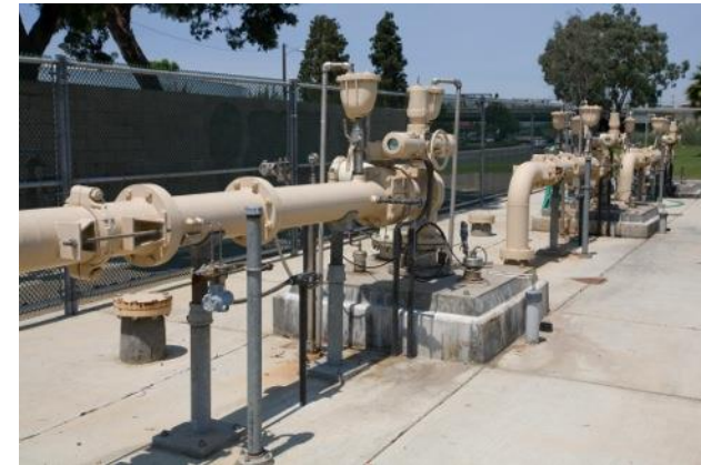
Typical injection well - OCWD
