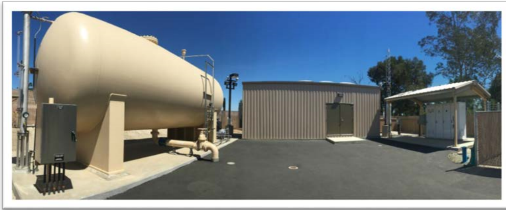
Photo 1 Part of the consolidation effort included new water infrastructure, such as a new water pump Station.
