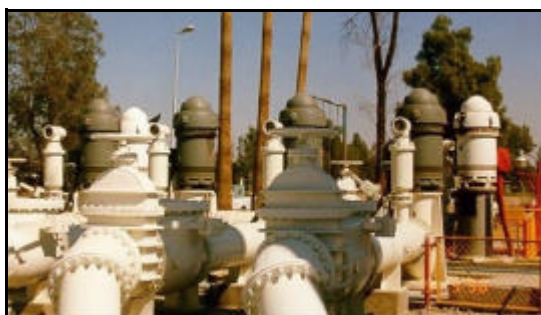
Figure 202 - Pumping Plant No. 1. The new pumps are shown in gray color (Jan 1998)
