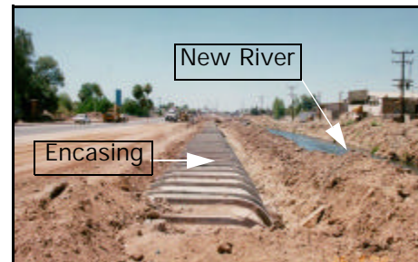
Figure 209 - New River by Pumping Plant No. 2 (Jun 1998)
