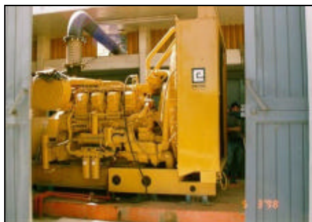
Figure 196 - Standby generator at Pumping Plant No. 1 (Mar 1998)
