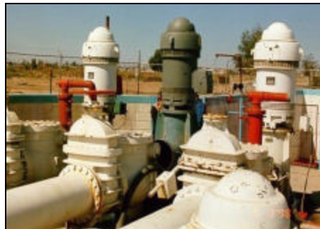
Figure 197 - Pumping Plant No. 3 (new pump in gray) (Mar 1998)
