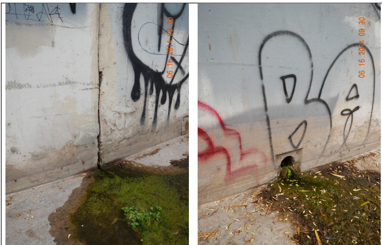
Figure 6-42. Photos of groundwater seepage into Franklin Creek. Photo Credit: Central Coast Water Board staff June 16, 2014.
