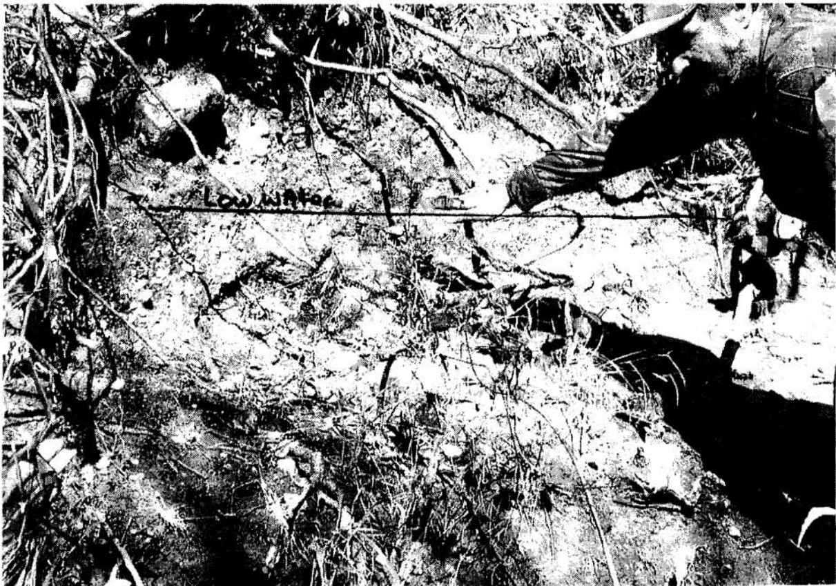
Figure 27. Accelerated Bank Degradation Due to Cut Bench in Previously Consolidated Bank Formation
