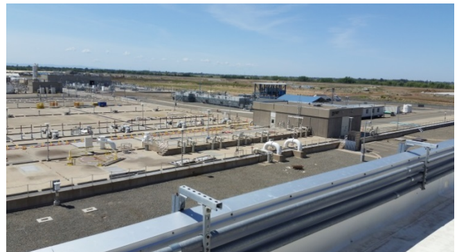
Sacramento Regional Wastewater Treatment Plant
