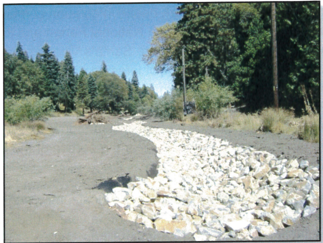
Photo 2: View looking northeast/downstream along constructed Hook Creek channel. Note that the view in this photo is the same as that in Photo 1.
