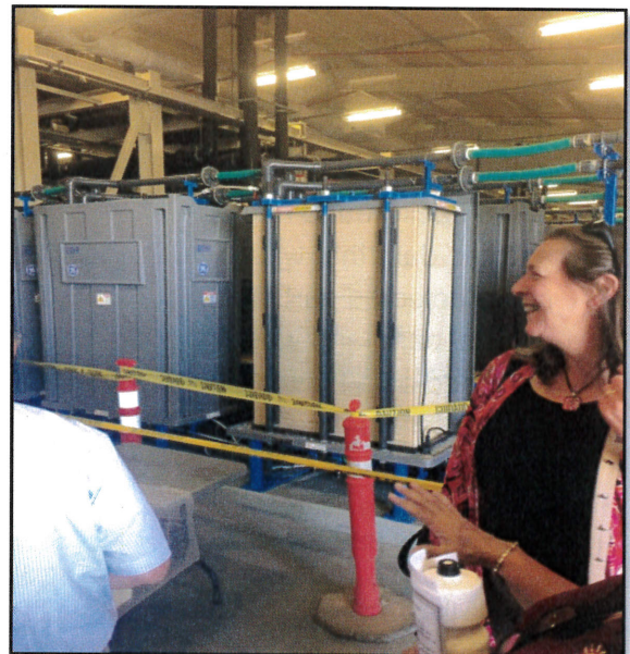
The electrodialysis membrane technology that is used in conjunction with reverse osmosis to treat supply water at the new Irwin Water Works. Employees can control the plant operations and the production wells from the state-of-the-art control room.
