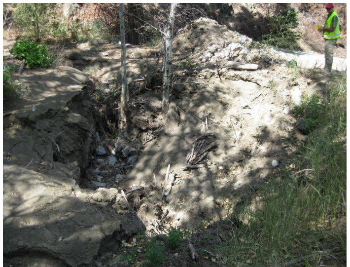
Culvert under Wolf Creek Road which was buried by the debris flow and subsequently caused flooding and erosion of the road bank and road shoulders
